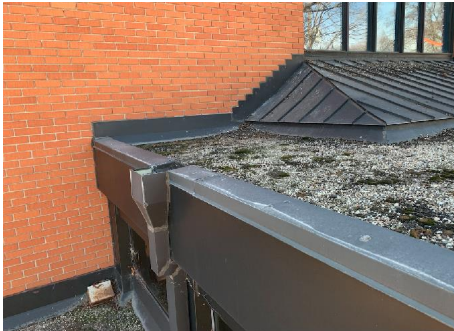
Fig. 11: Roof-B: Save splash pans for re-use. Modify & seal new reglet flashing(s) as required.
