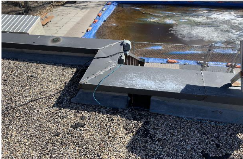
Fig. 8: Roof-A: Exterior electrical by City of Winnipeg. Parapet tops to be re-sloped back to roof a min. of 2%.
