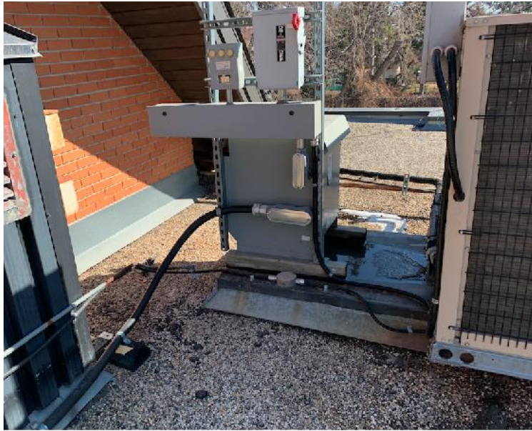
Fig. 7: Roof-A: Modify & raise platform curb including electrical & mechanical to facilitate min. 8" above new roof height.
