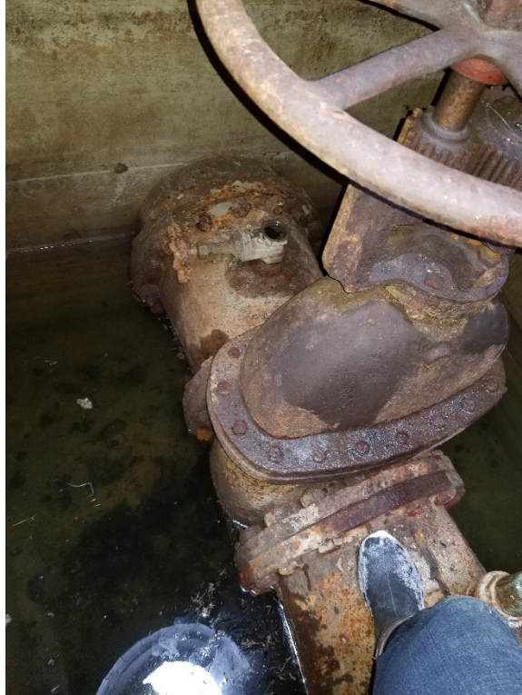
Site 10 – Existing 50 mm air valve in south chamber, looking north.
