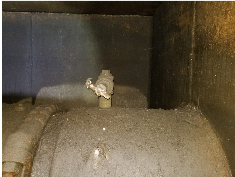
Site 7 – Existing West 50 mm Gate Valve, looking South from bottom of ladder.
