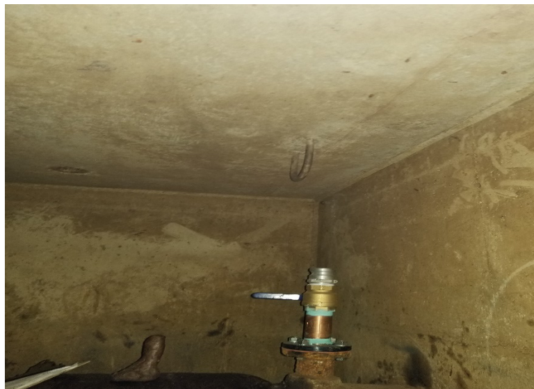
Site 11 – Existing 50 mm air valve and roof slab in chamber located west of McPhillips Street.
