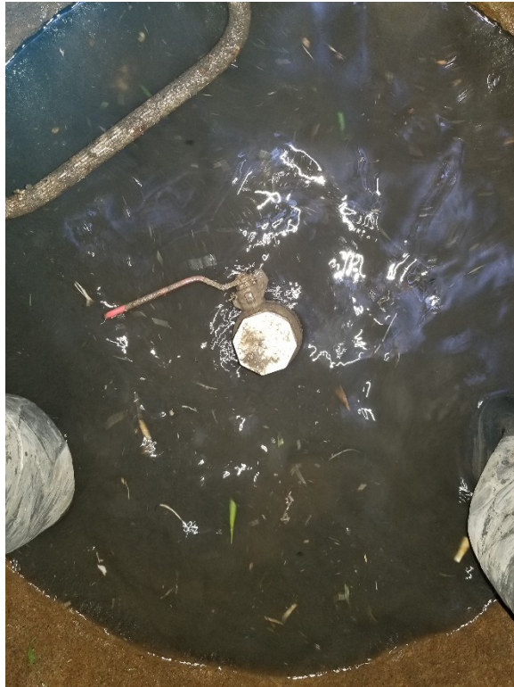
Site 9 – Existing air release valve in existing 750 manhole.
