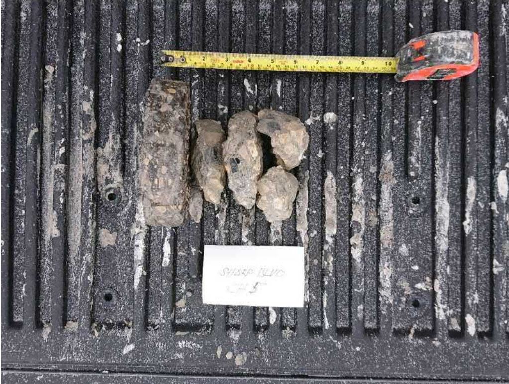
Photograph 5: Core Hole CH20-05 – Concrete partially recovered
