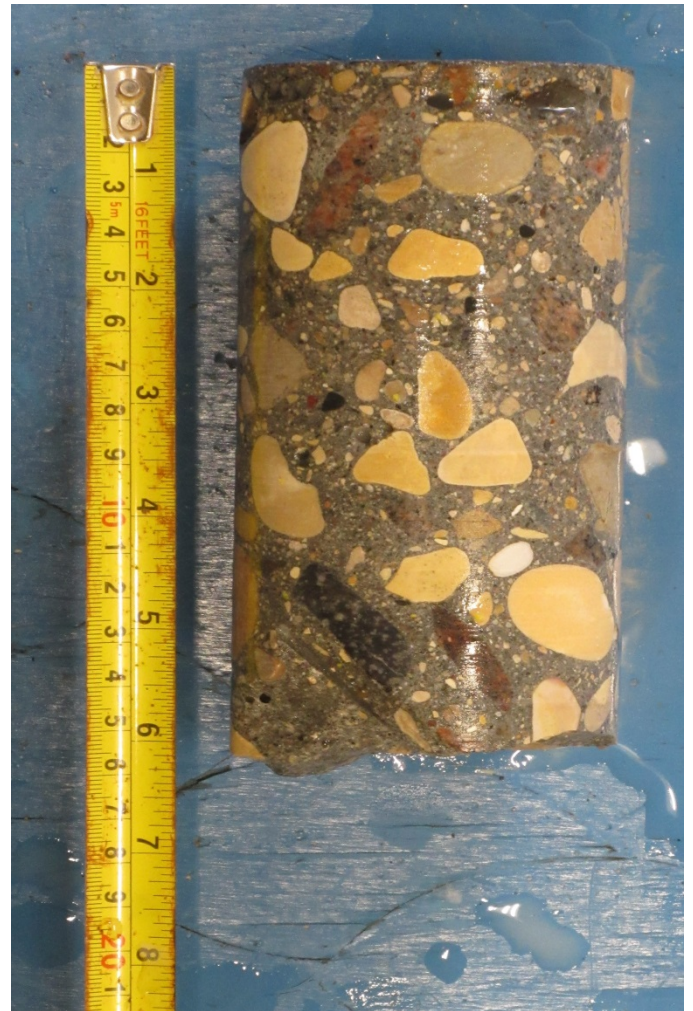
Figure 26 – Core no. A6, west abutment
