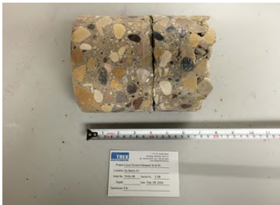
Photo 8: Pavement Core Sample at Test Hole TH16-08 (core had to be broken off during coring)
