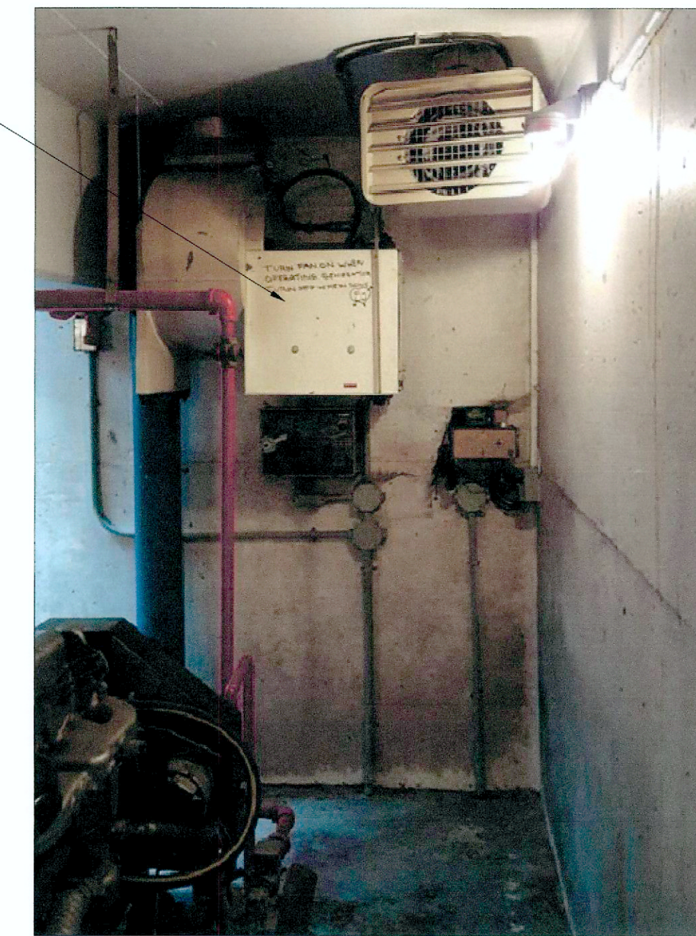
EXISTING STATION EXHAUST FAN
