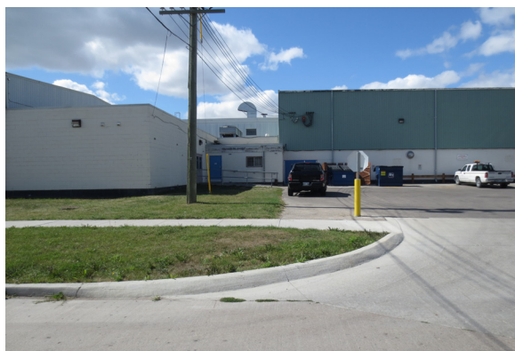
Main distribution to the building and Hydro pole
