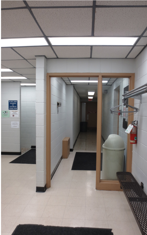
Corridor to weight room. The door has been removed from the steel frame
