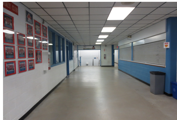
Above: Waiting area with canteen on the right. Windows on the left have view to the hockey arena.
