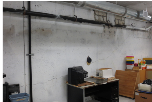
Crack in the basement wall
