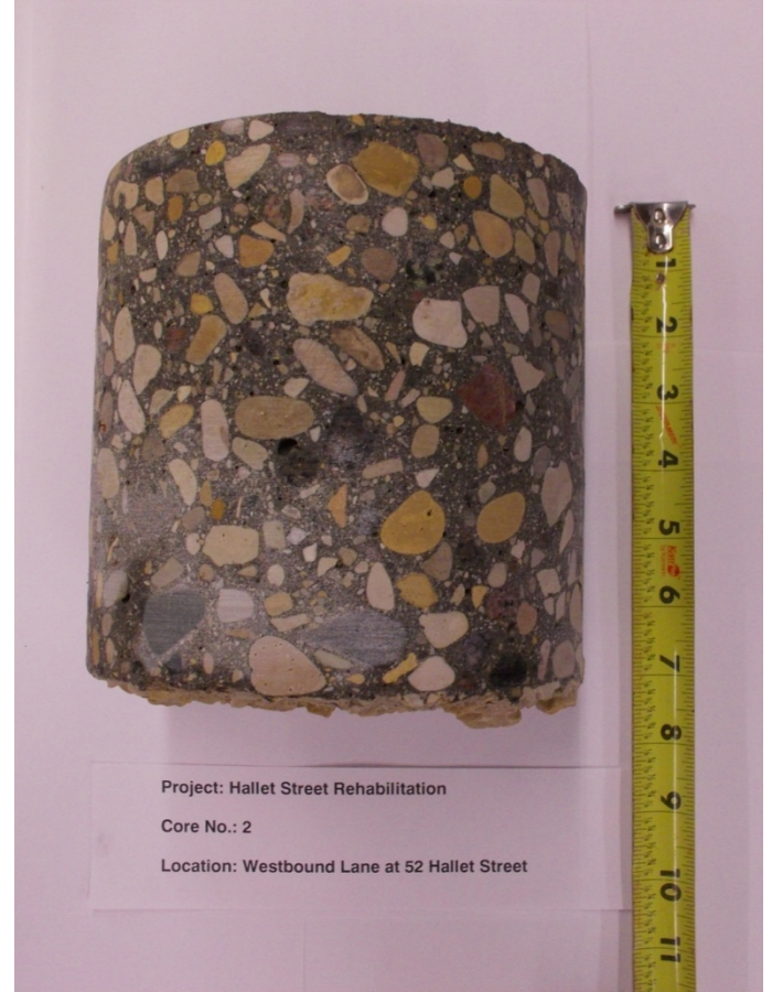
Photo 2: C02: Westbound lane at 52 Hallet Street, 1.0 m from curb
