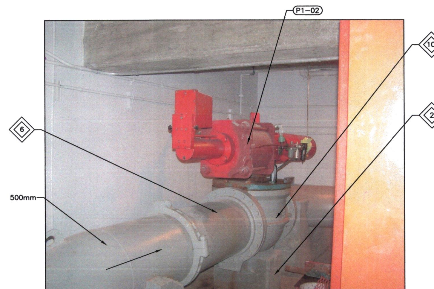
8 SHUTDOWN 7 - CONTROL VALVE P1-02 M2
