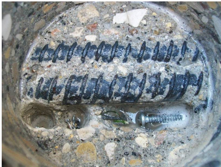
CONDITION OF EXPOSED REBAR ON THE SOUTHBOUND LANE
