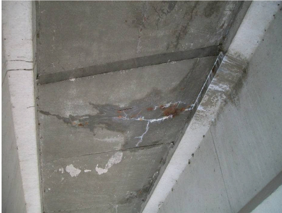
EFFLORESCENCE OBSERVED ON THE UNDERSIDE OF THE EAST SIDE OF THE NORTHBOUND BRIDGE
