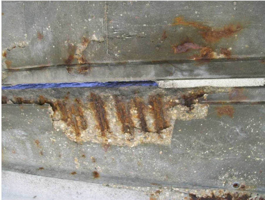
ISOLATED CORROSION AND DELAMINATION OBSERVED ON THE EAST SIDE OF THE SOUTHBOUND BRIDGE
