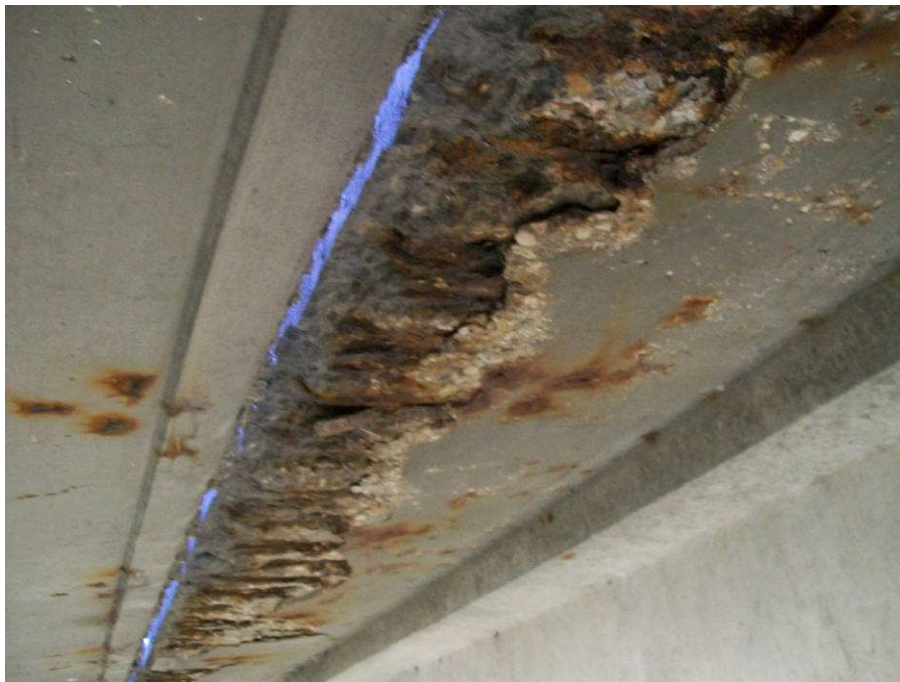
HEAVY CORROSION AND DELAMINATION OBSERVED ON THE WEST SIDE OF THE NORTHBOUND BRIDGE
