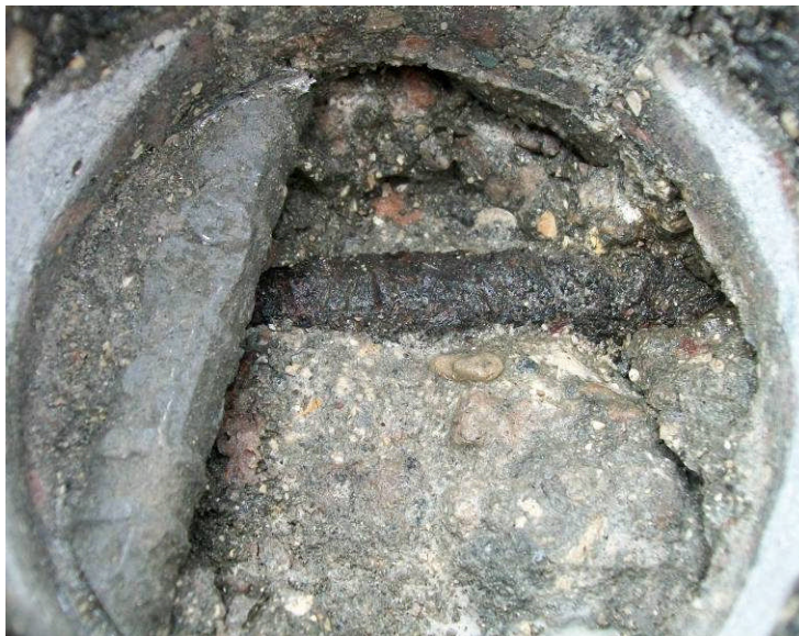
CONDITION OF EXPOSED REBAR ON THE NORTHBOUND LANE
