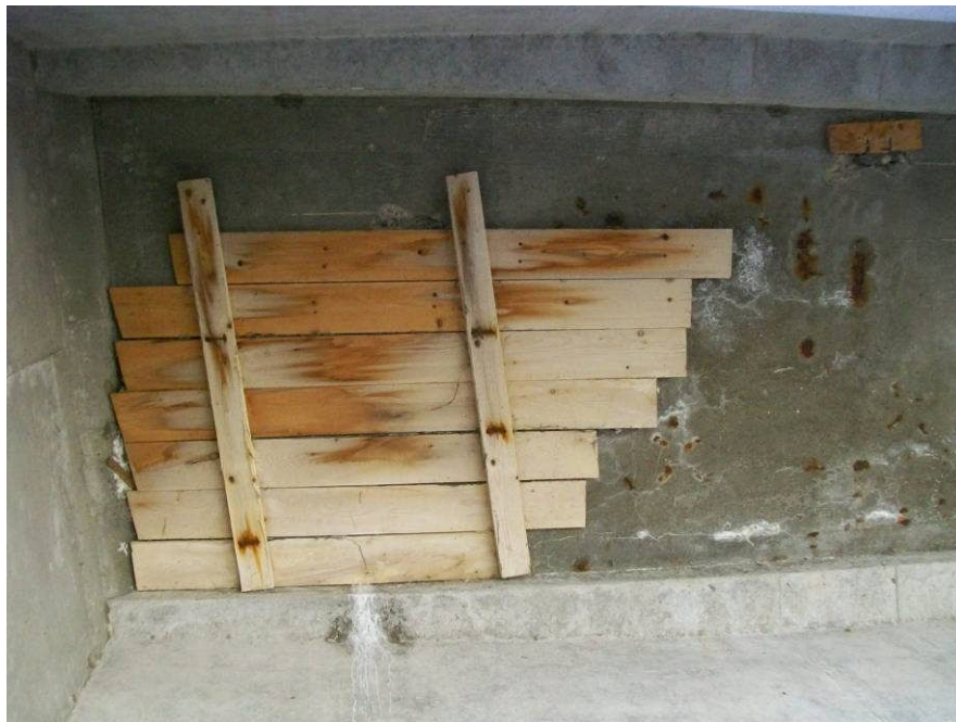
EVIDENCE OF PREVIOUS FULL DEPTH REPAIR
