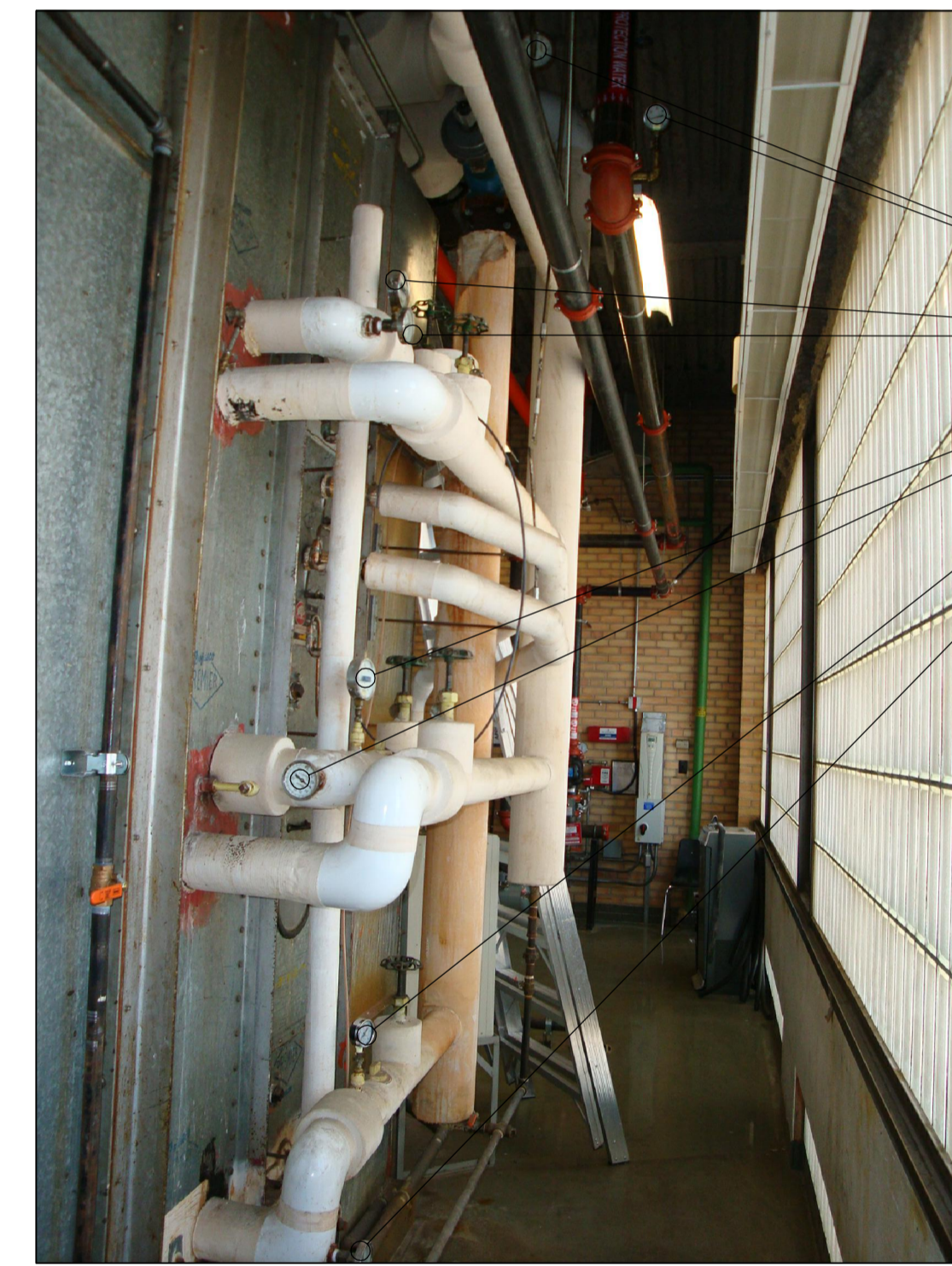
PHOTO A SCALE: NTS COLD DECK CHILLED WATER PIPING
