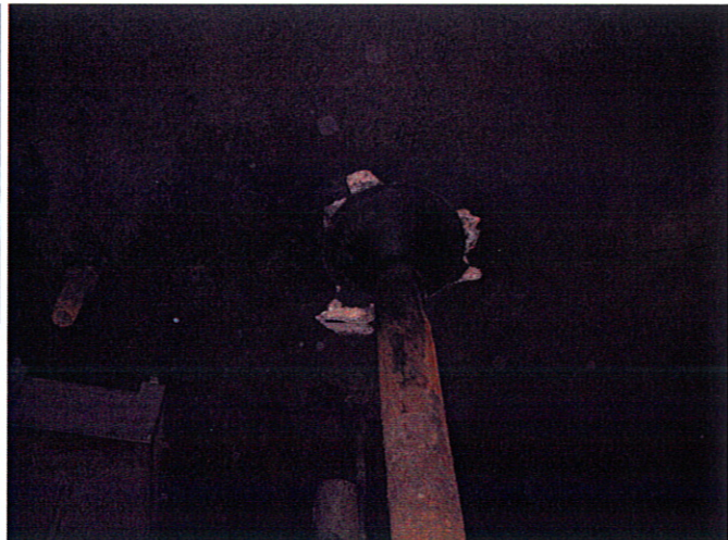
Photo 4: Fallen pieces of roof material around column capitals.
