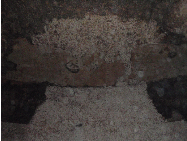
Scraped Section of Ceiling
