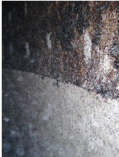
Levels 4 and 5, with Scraped Spots for Corrosion Potential Measurements
