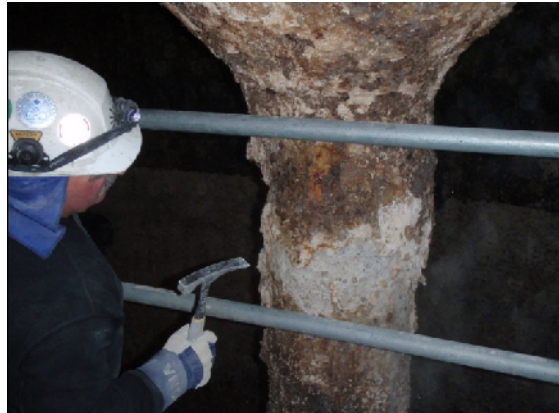
Ring Scraped on Column
