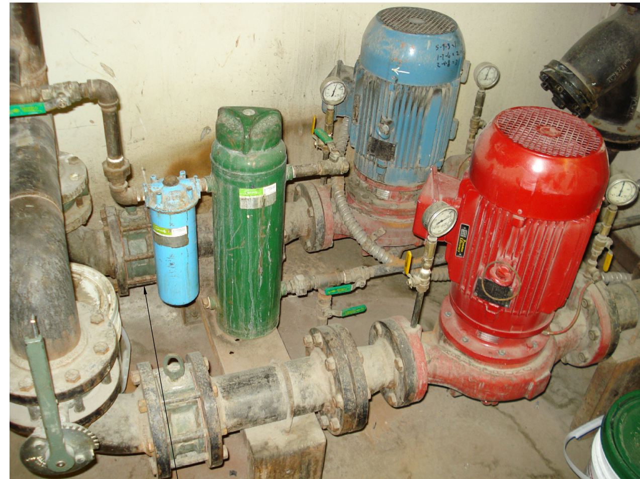
REMOVE AND REPLACE DEFECTIVE CHECK VALVE
