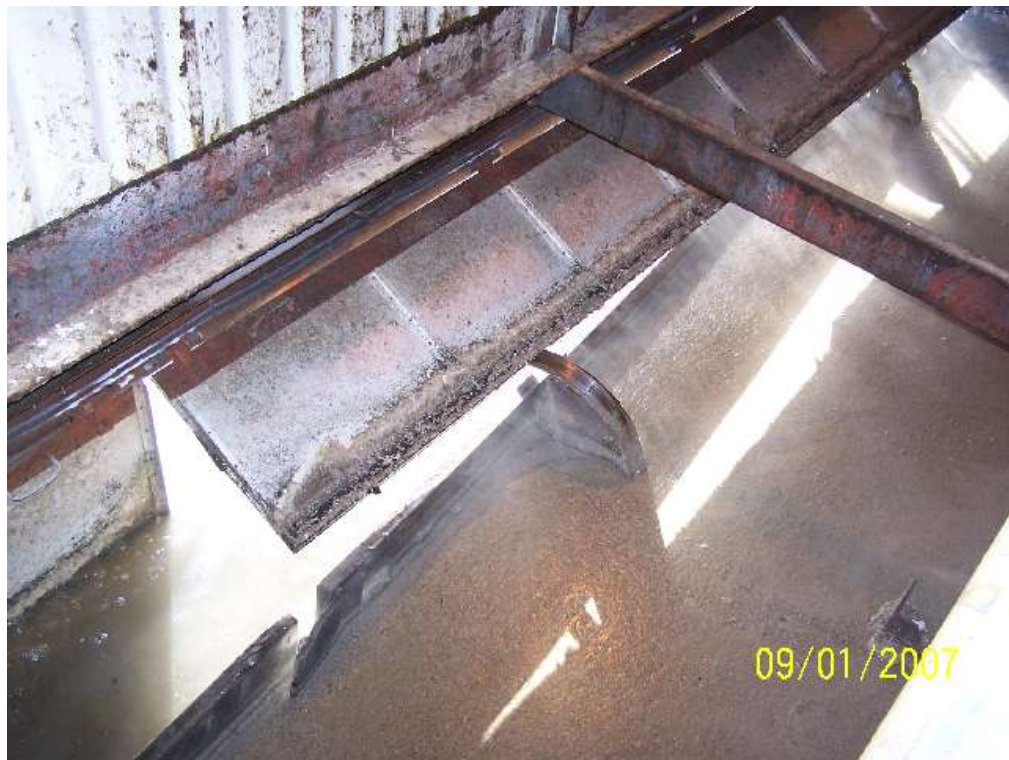
Photo 3-16 Walkway Enclosure Hinged Scum Blade Access Panels
