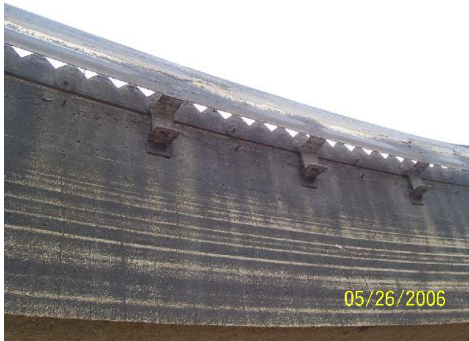
Photo 3-3 Effluent Weir & Scum Baffle
