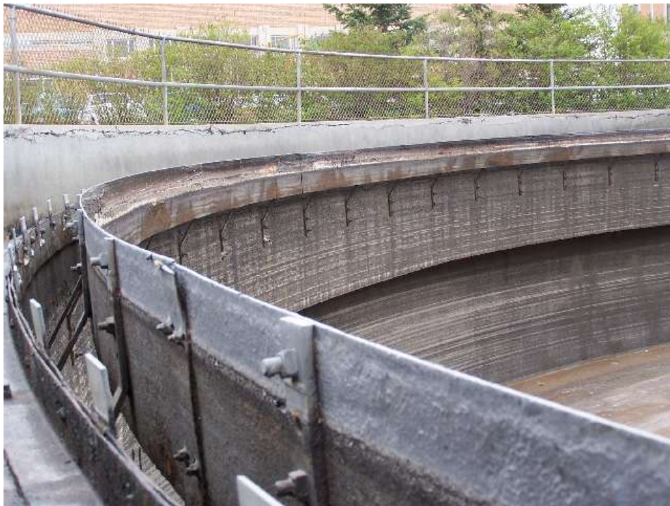
Photo 2-2 Effluent Weir & Scum Baffle
