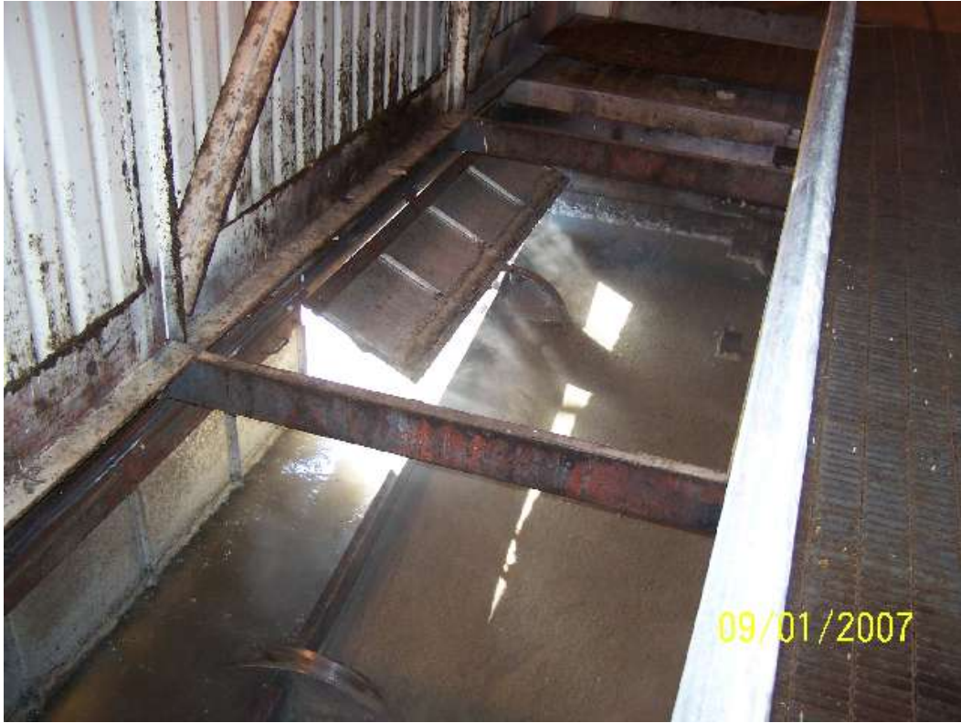
Photo 3-17 Walkway Enclosure Hinged Scum Blade Access Panels
