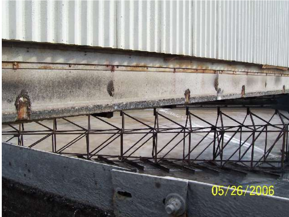
Photo 3-7 Walkway Enclosure Hinged Scum Blade Access Panels
