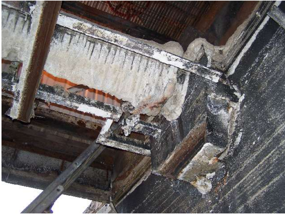
Photo 2-1 Scum Trough Discharge Box
