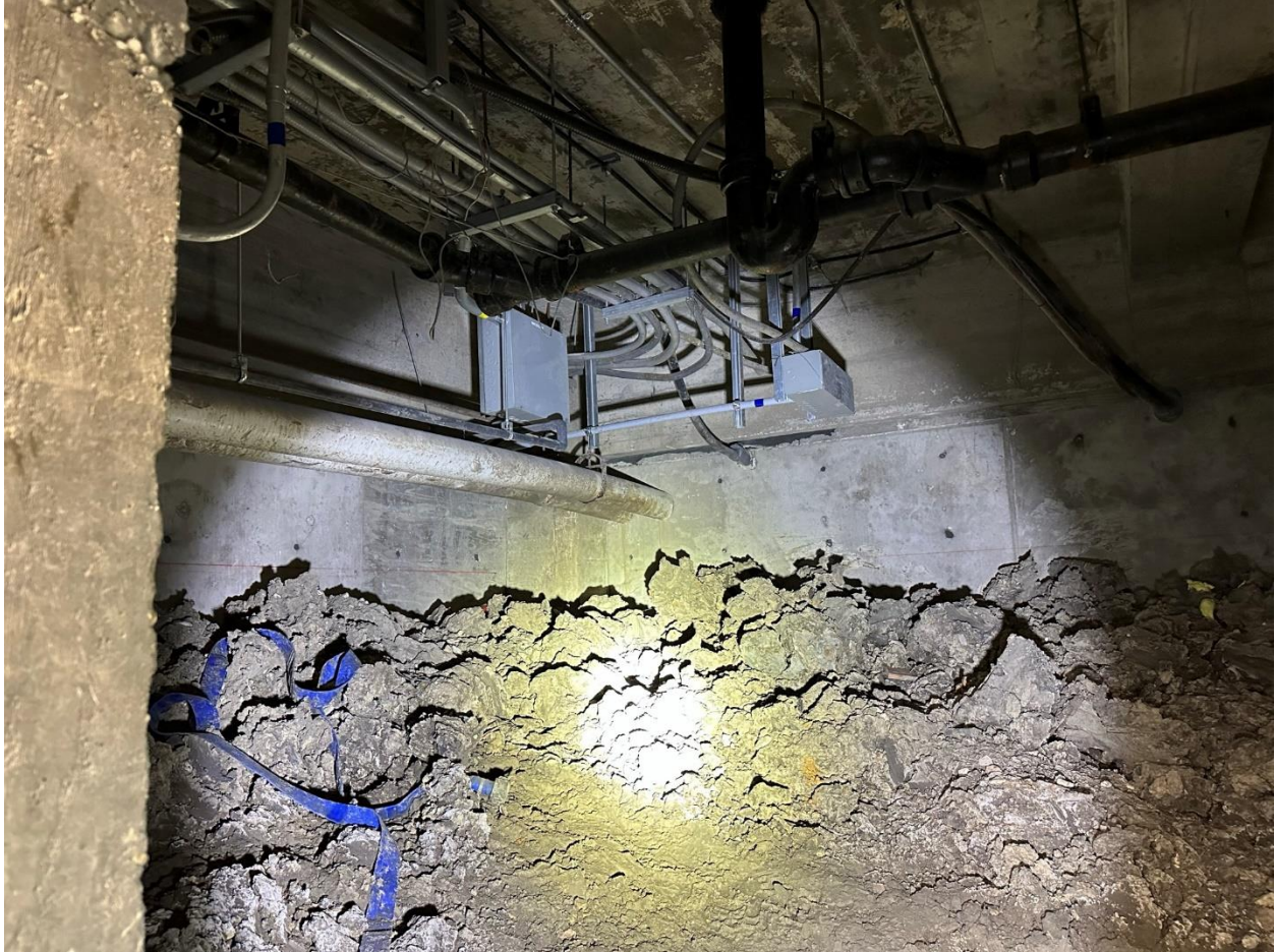
Figure 7: Southeast corner of crawlspace showing existing cooling tower pipes penetrating the grade beam extension.
