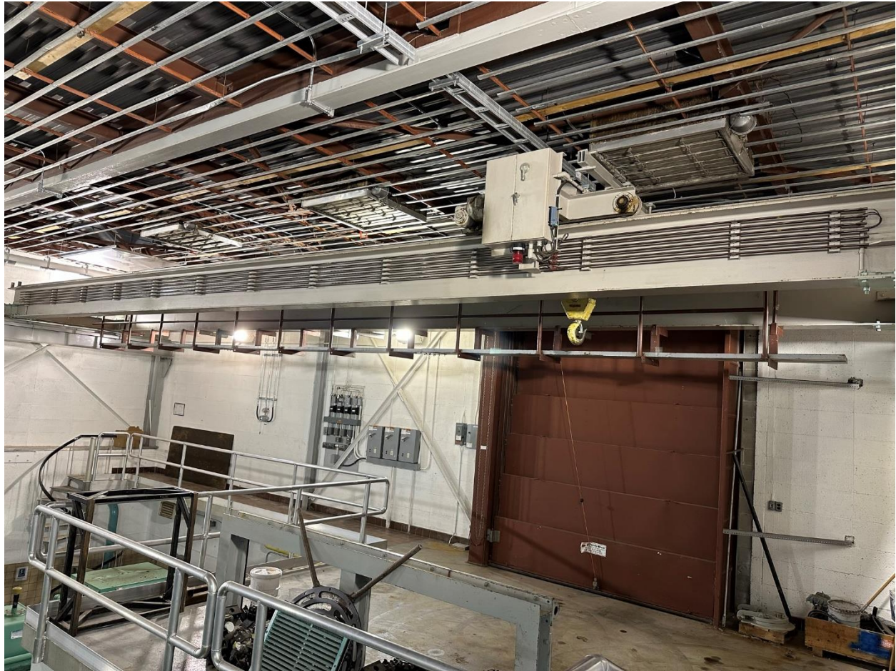
Figure 3: Looking west showing three existing exhaust fan dampers (ceiling), and existing starters, wiring, conduits, pneumatic piping, and control (wall).
