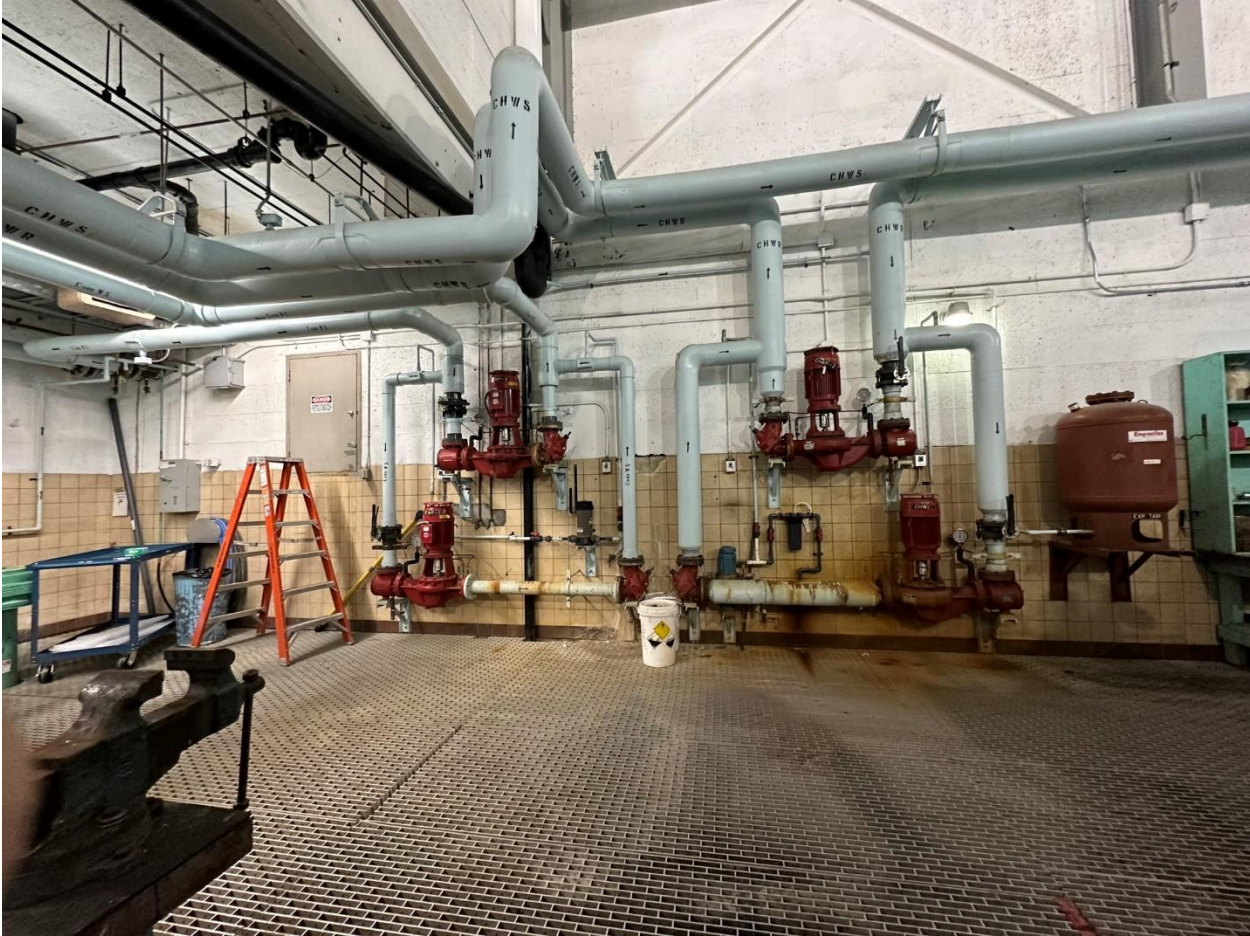
Figure 12: Looking south showing existing chilled water pumps, cooling tower pumps, and expansion tank.
