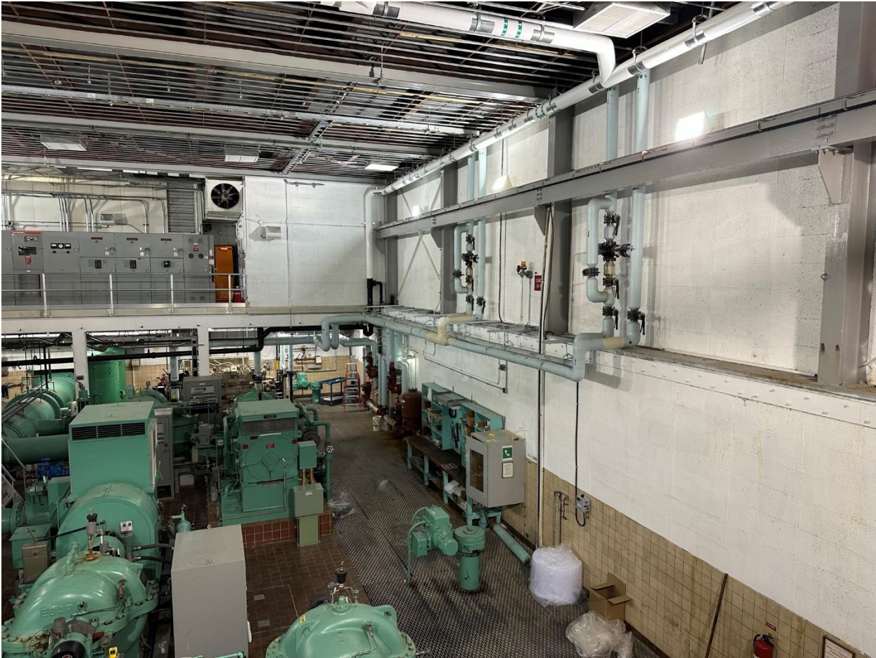
Figure 13: Looking east showing existing chilled water piping up to two rooftop air handling units.
