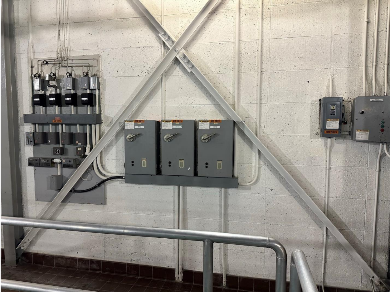
Figure 5: Existing starters, wiring, conduits, pneumatic piping, and control for three exhaust fans.
