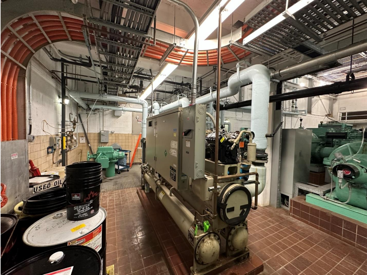
Figure 11: Existing indoor chiller, looking southwest.
