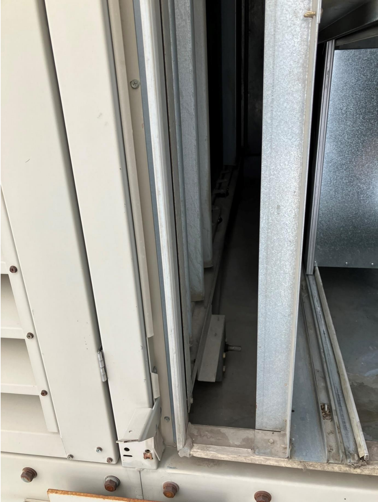
Figure 2: AHU-2 damper manual actuator.
