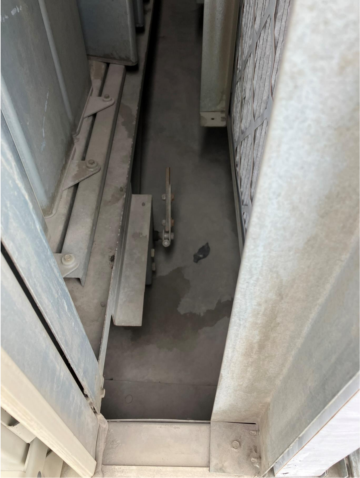
Figure 1: AHU-1 damper manual actuator.
