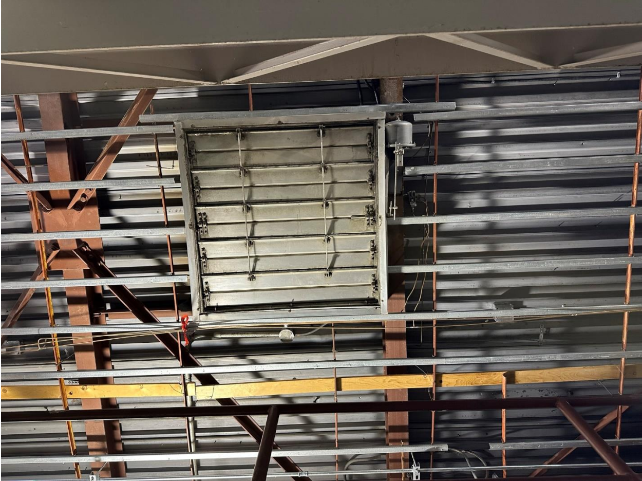
Figure 4: Existing exhaust fan damper and actuator - typical of three.
