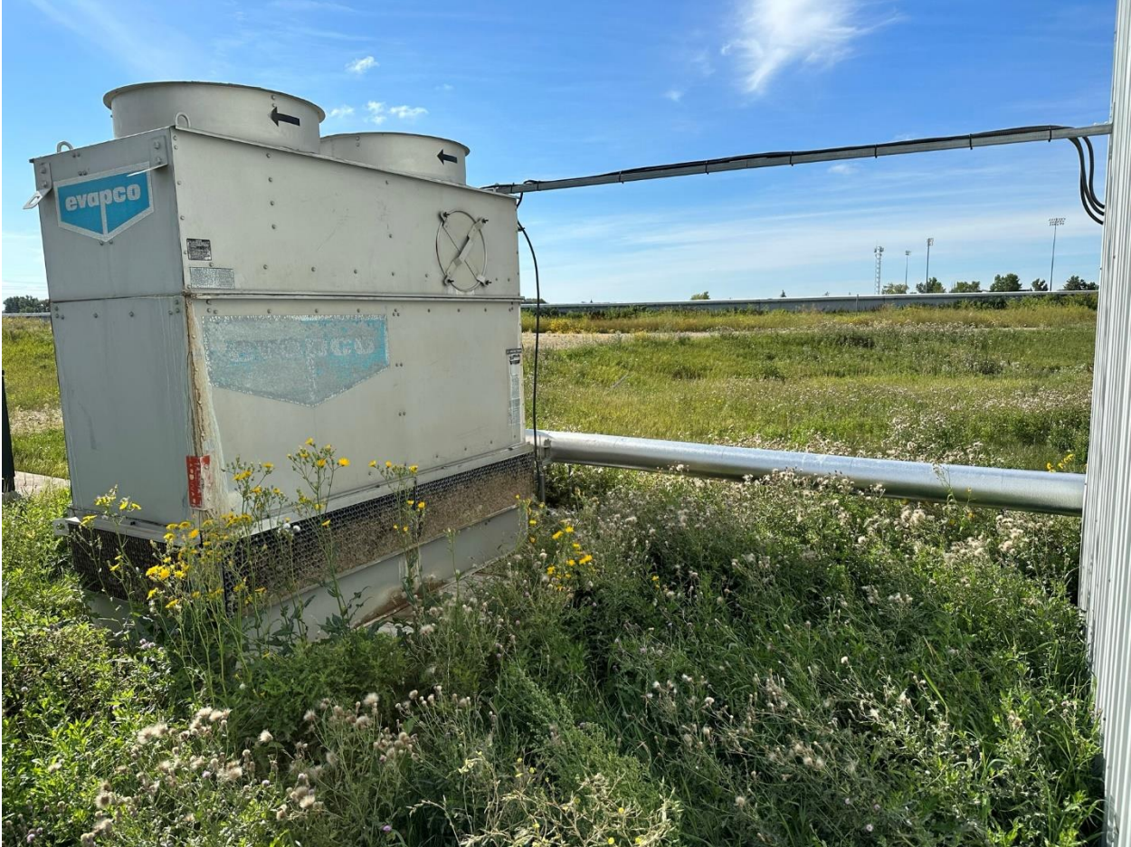
Figure 16: Existing cooling tower.
