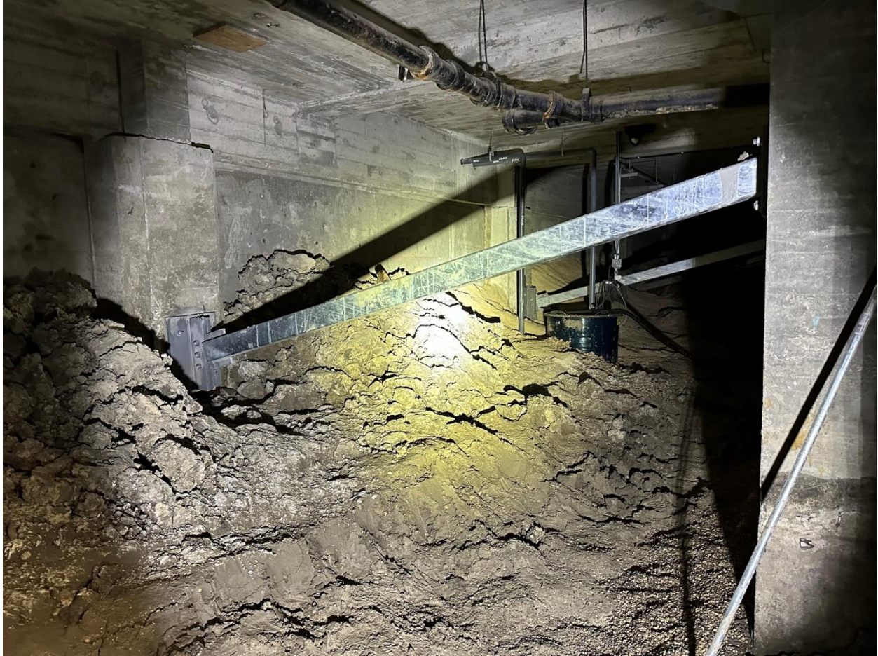
Figure 8: Looking west in crawlspace showing existing sump basin and piping penetrating original grade beam.
