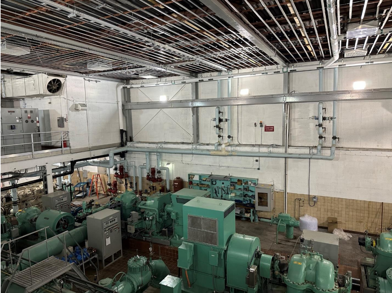
Figure 14: Looking south showing existing chilled water piping up to two rooftop air handling units.
