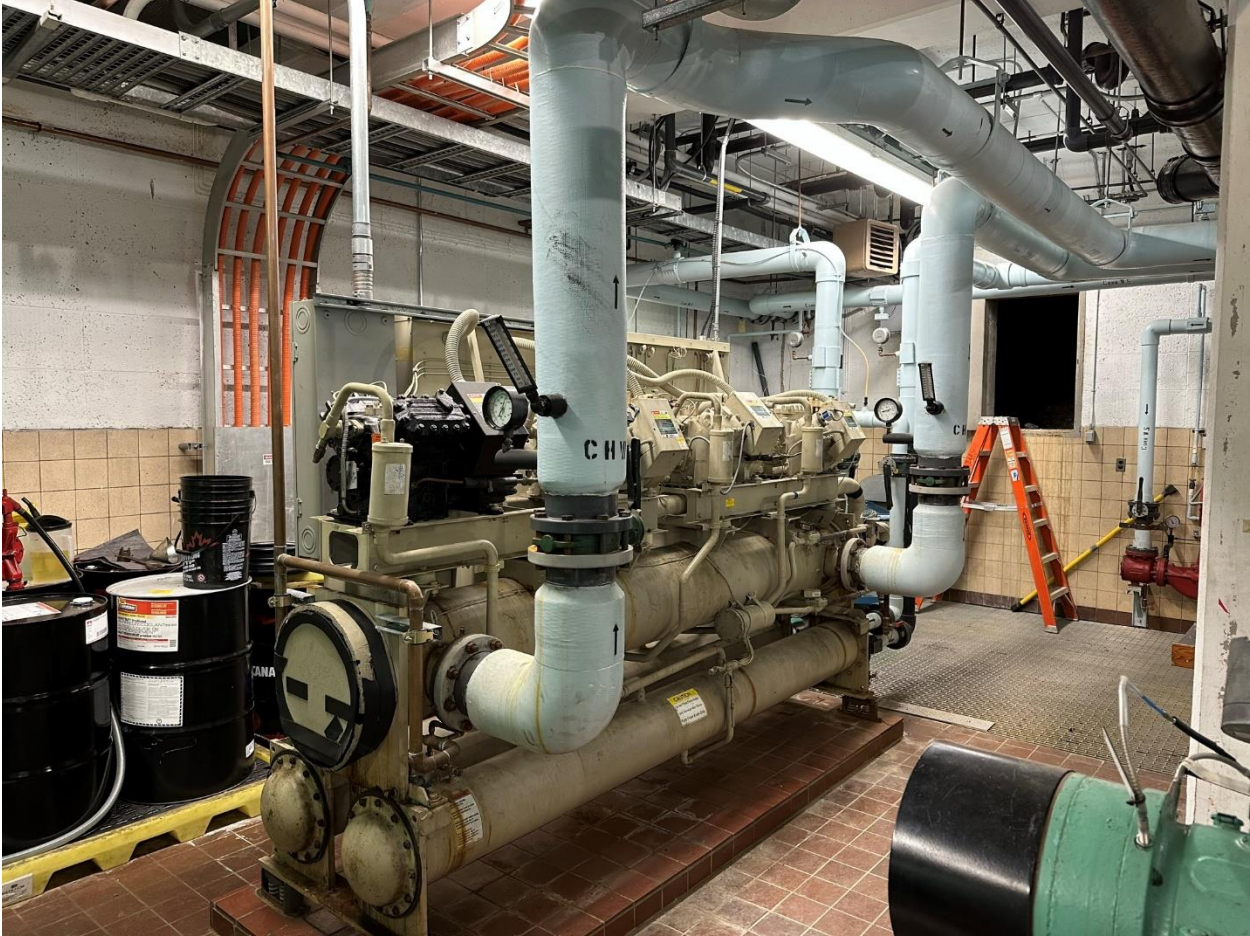
Figure 10: Existing indoor chiller, looking southeast.
