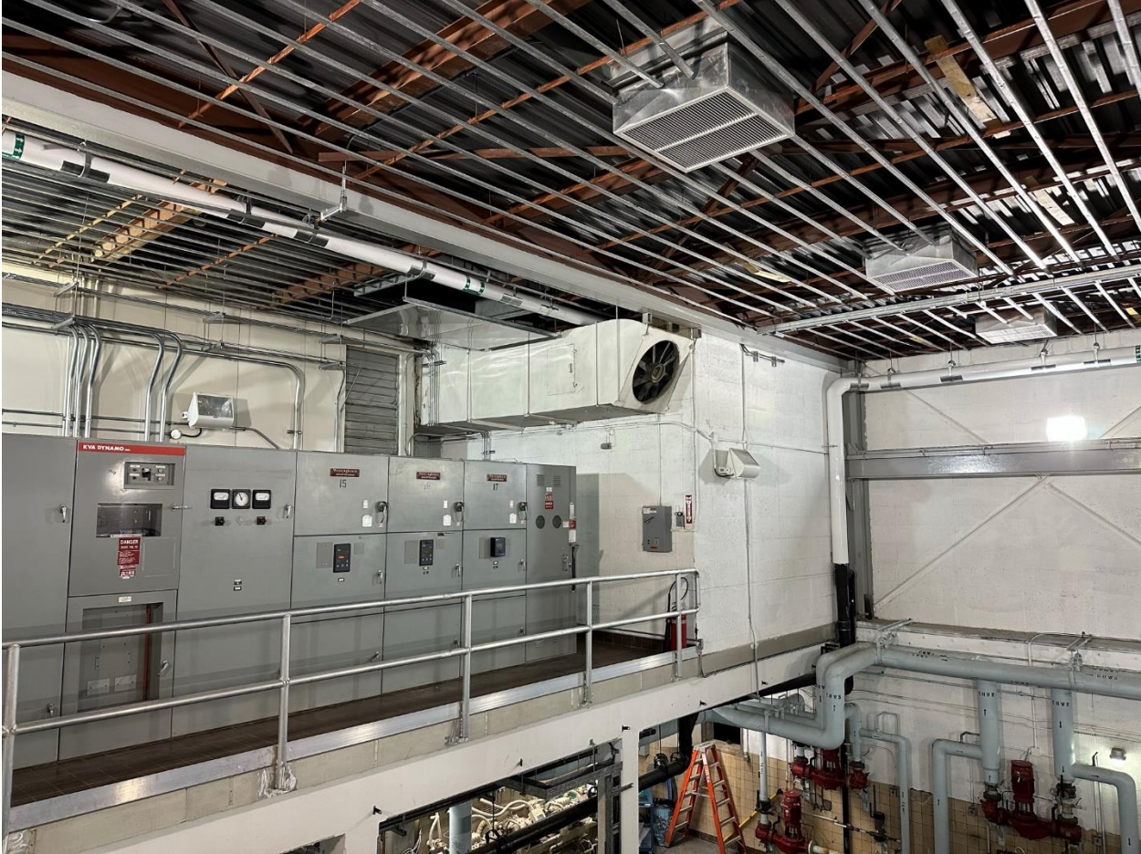
Figure 6: Looking east showing existing supply air fan.
