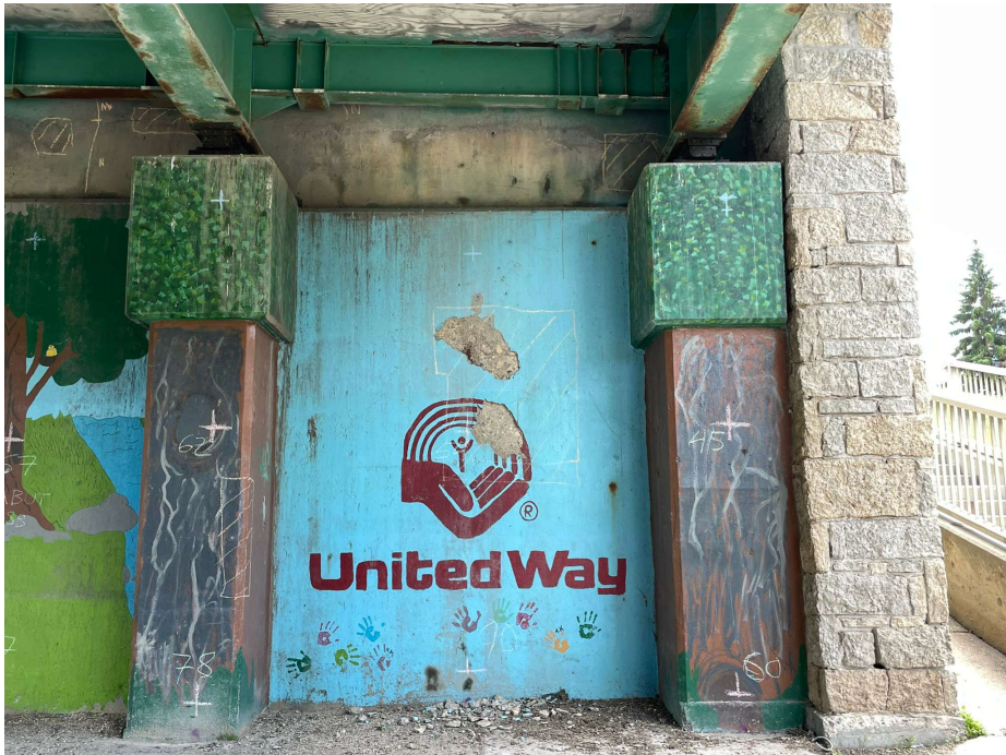
Photo 26 - South abutment wall, SB, between Column 9-10, large delamination and spalling
