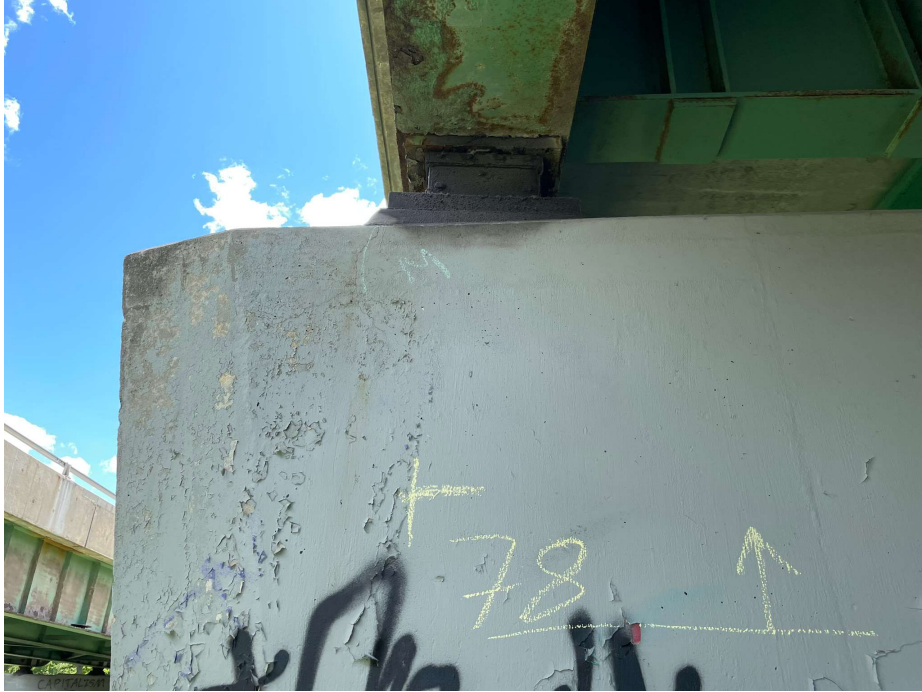
Photo 49 - Typical medium vertical cracks under bearing locations
