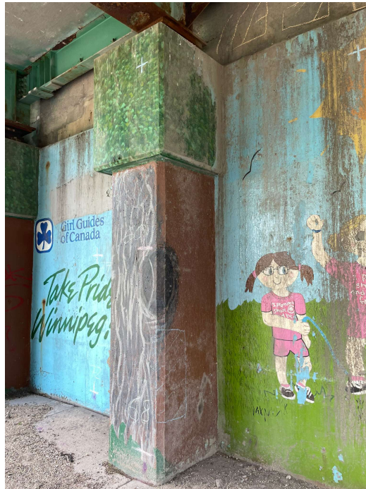
Photo 19 - South abutment wall, NB, at Column 2, localized delamination
