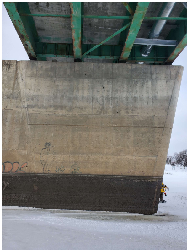
Photo 26 - Pier 6 South Face East Section 13 of 22
