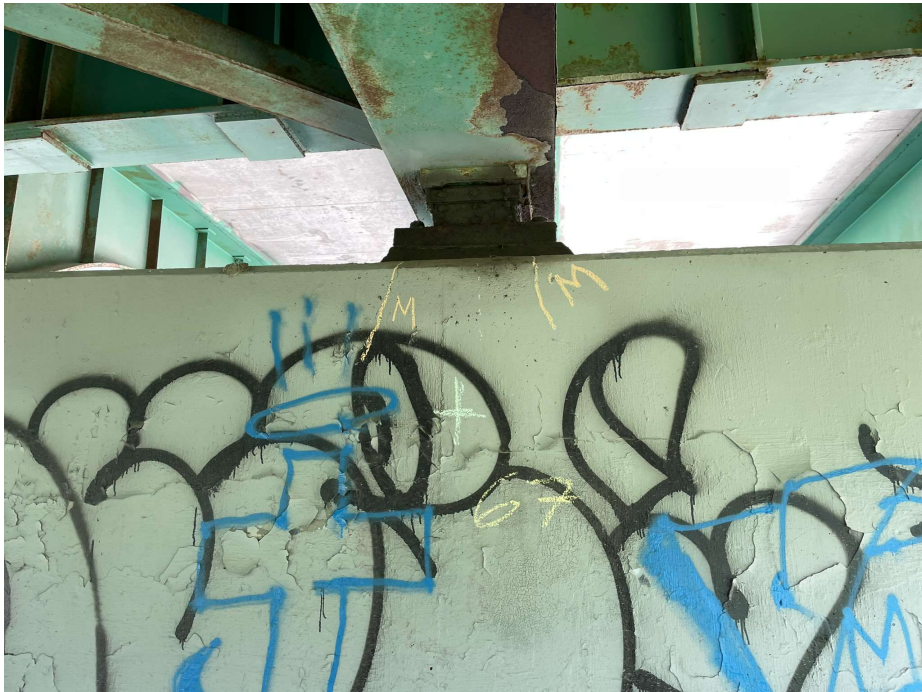
Photo 50 - Typical medium vertical cracks under bearing locations, additional view
