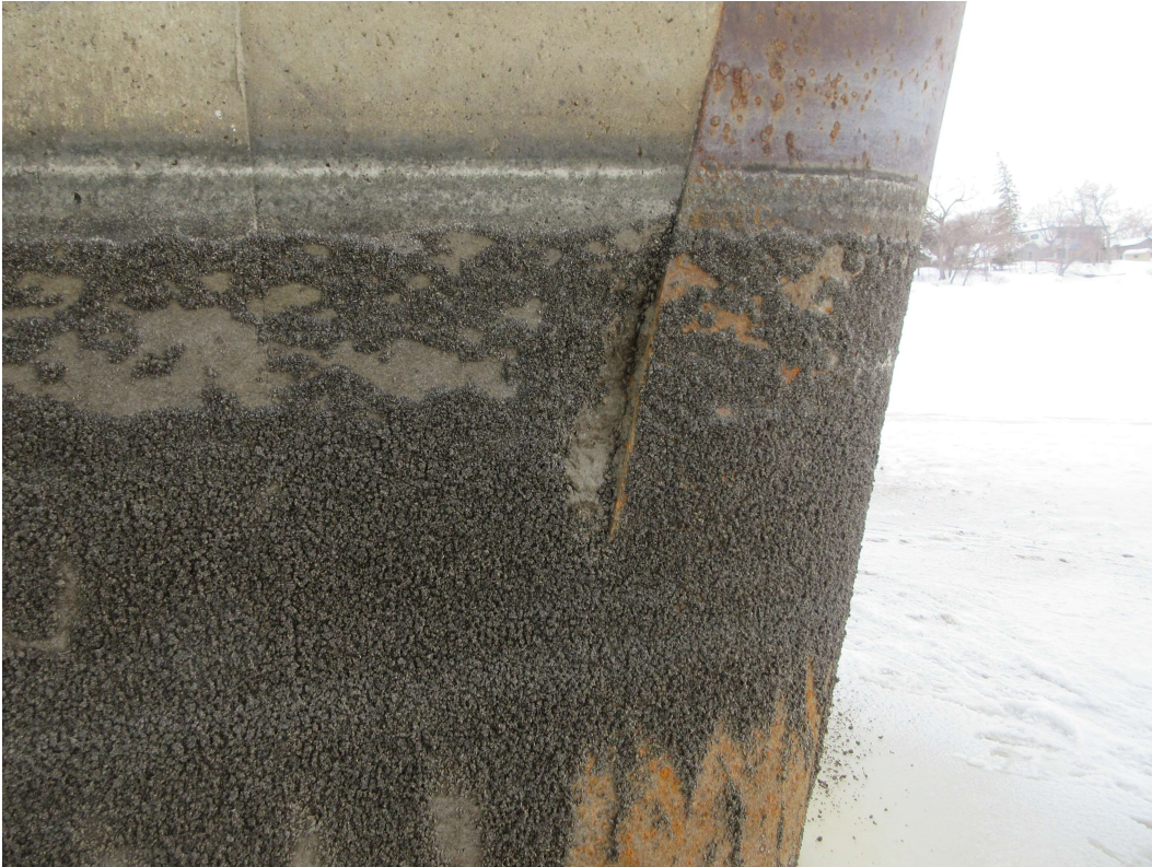
Photo 33 - Pier 4 North Face Spall
