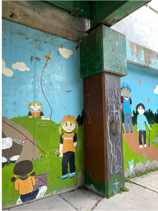
Photo 21 - South abutment wall, NB, at Column 4, localized small delaminations
