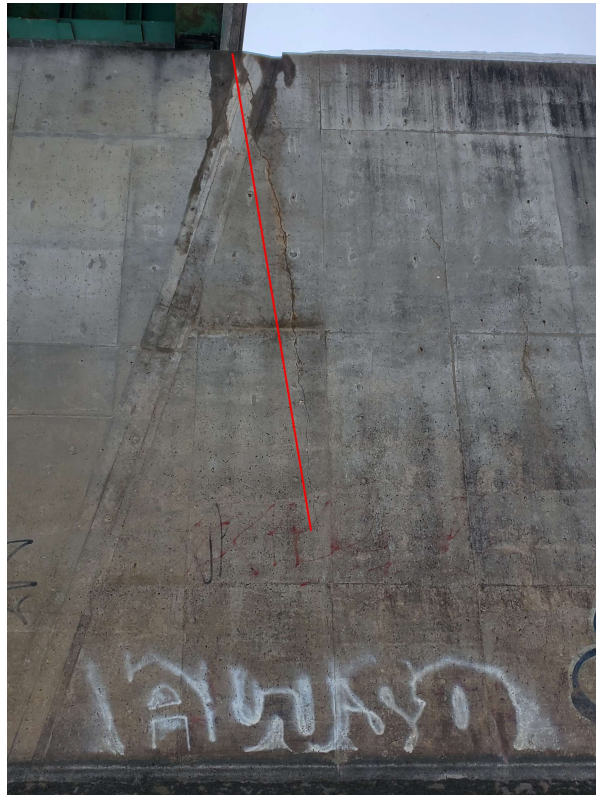
Photo 31 - Pier 4 North Face Wide Crack
