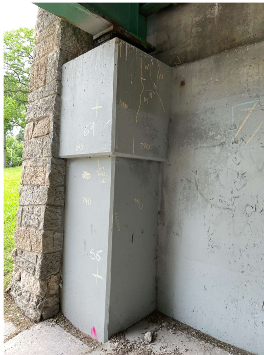
Photo 04 - North abutment NB, Column 1 cap, narrow to wide cracking
