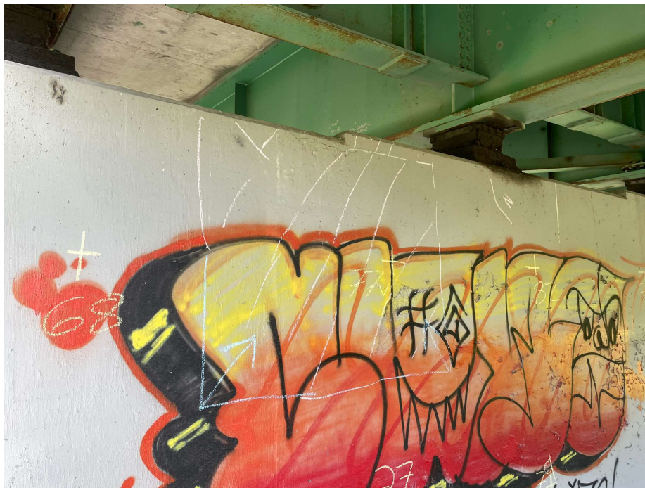
Photo 42 - Pier 7 SB, south face, localized delamination near west end at top of pier
