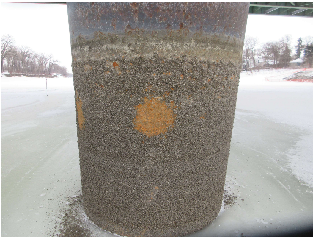
Photo 38 - Medium Pitting on Pier 5 Nosing 19 of 22
