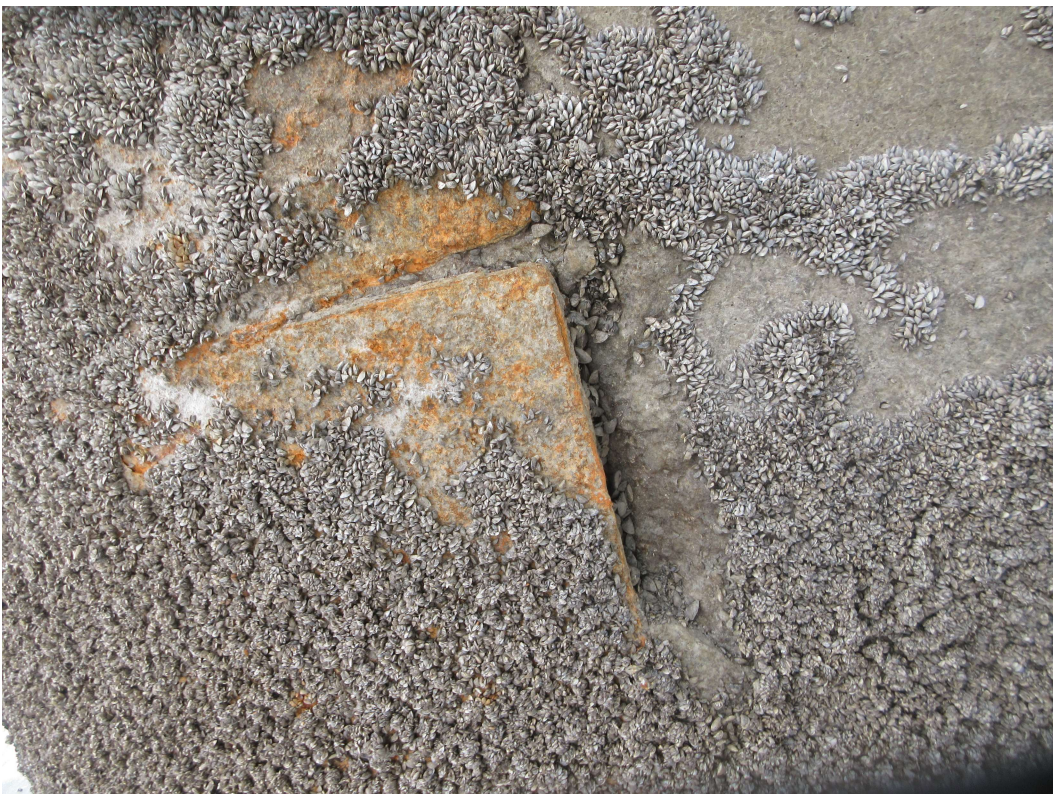
Photo 40 - Pier 5 South Face Spall 20 of 22
