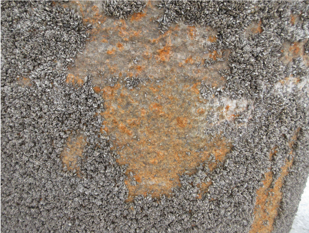
Photo 35 - Medium to Severe Pitting on Pier 4 Nosing, Close up View
