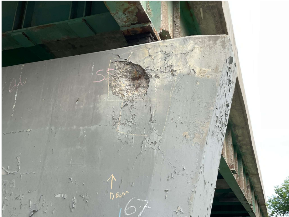
Photo 31 - Pier 1 NB, north face, localized spall at top of pier near west end
