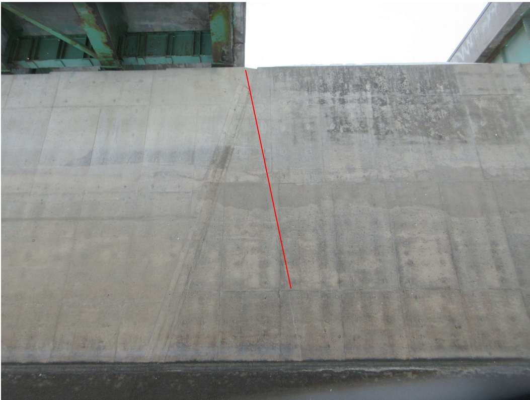
Photo 36 - Pier 5 North Face Medium Crack 18 of 22
