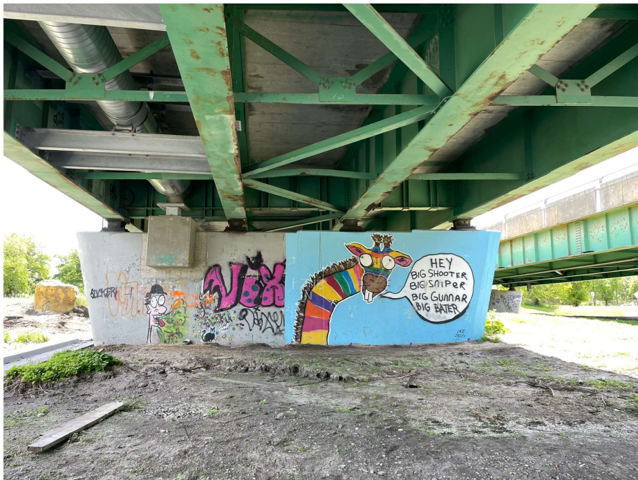
Photo 38 - Pier 7 NB, north face, note recent modification from forced main sewer
