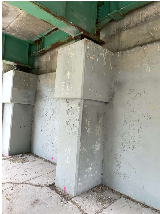
Photo 07 - North abutment NB, Column 2 cap east face, medium to wide cracking
