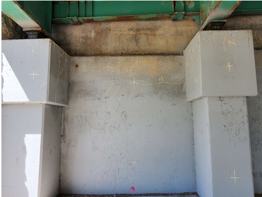
Photo 05 - North abutment wall, between Column 1-2, medium horizontal crack and localized delamination
