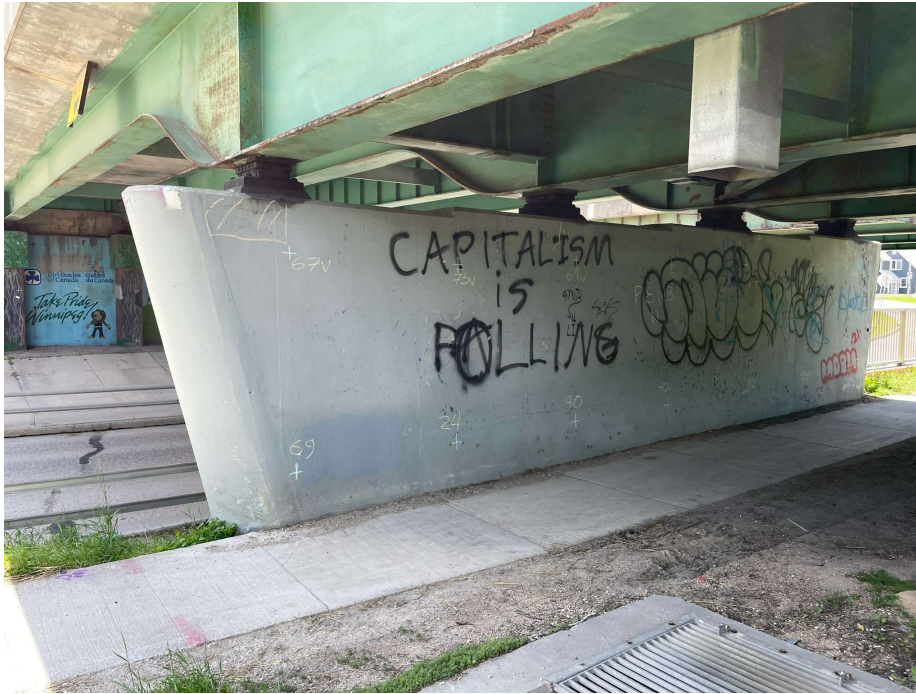
Photo 47 - Pier 8 NB, north face, localized delamination under eastmost bearing
