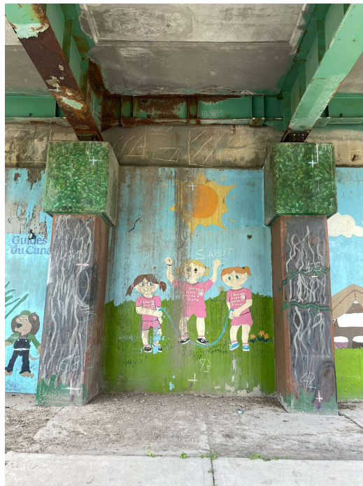
Photo 20 - South abutment wall, NB, between Columns 2 and 3, joint leakage / staining, and large areas of delamination on ballast wall
