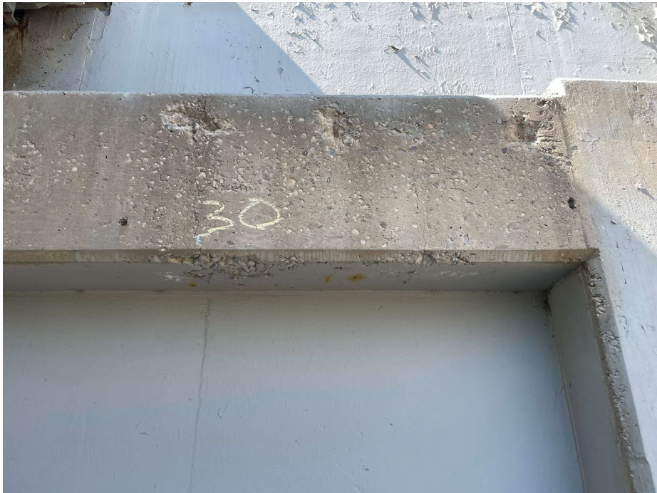
Photo 14 - North ballast wall – localized delamination at east end of SB lanes
