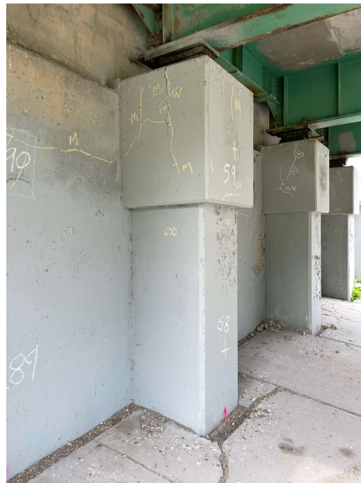
Photo 06 - North abutment NB, Column 2 cap west face, medium to wide cracking
