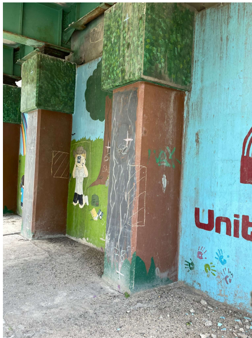
Photo 24 - South abutment wall, SB, between Column 8 and 9, localized delaminations on column bottoms
