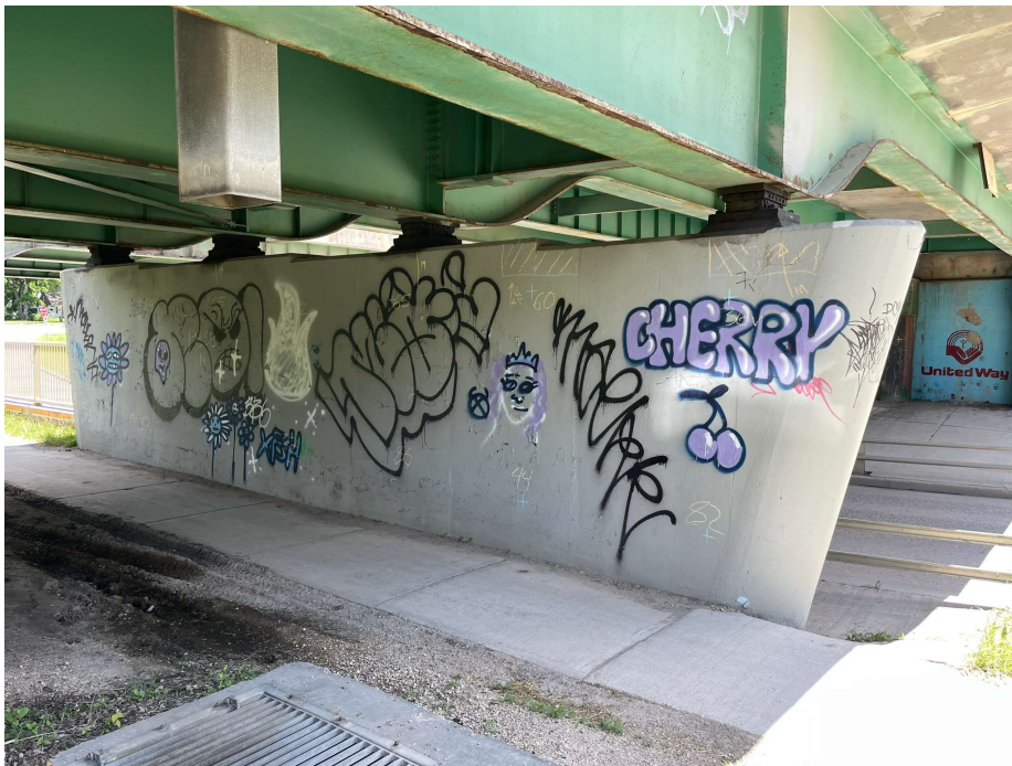
Photo 48 - Pier 8 SB, north face, localized small delaminations near top of pier at west end and at 1st bearing seat step from West end
