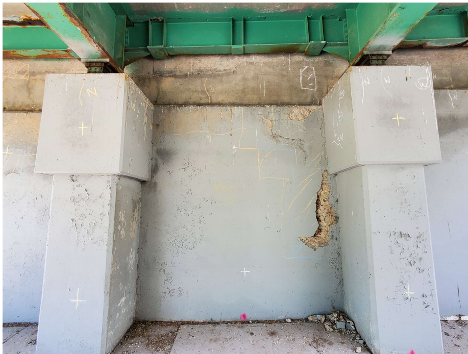
Photo 08 - North abutment wall, between Column 2-3, large delaminations and spalling
