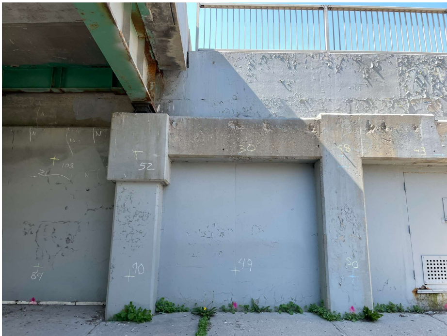
Photo 10 - North abutment wall between NB and SB – localized spalls, light scaling, and medium honeycomb on cap beam between Column 4 – 6
