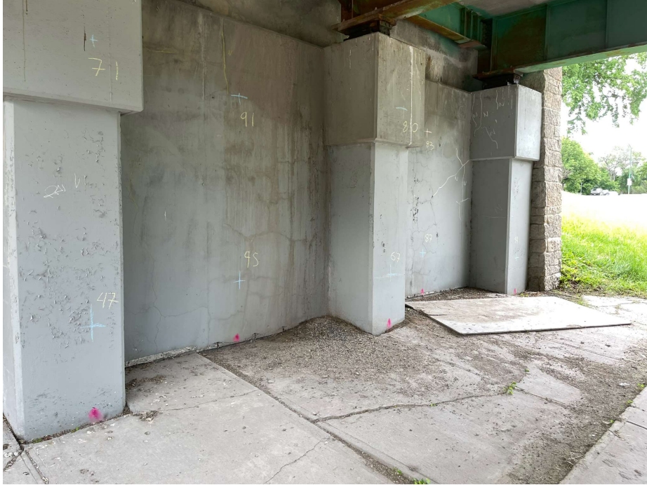
Photo 13 - North abutment, Column 8-10, narrow vertical and horizontal cracking on abutment wall refacing
