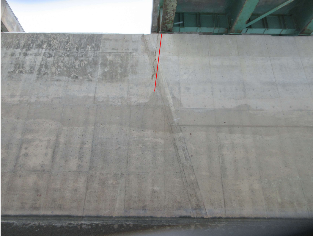
Photo 37 - Pier 5 North Face Medium Crack
