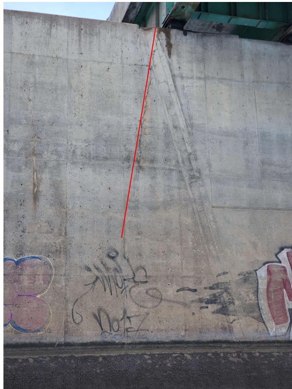
Photo 32 - Pier 4 South Face Medium Crack 16 of 22
