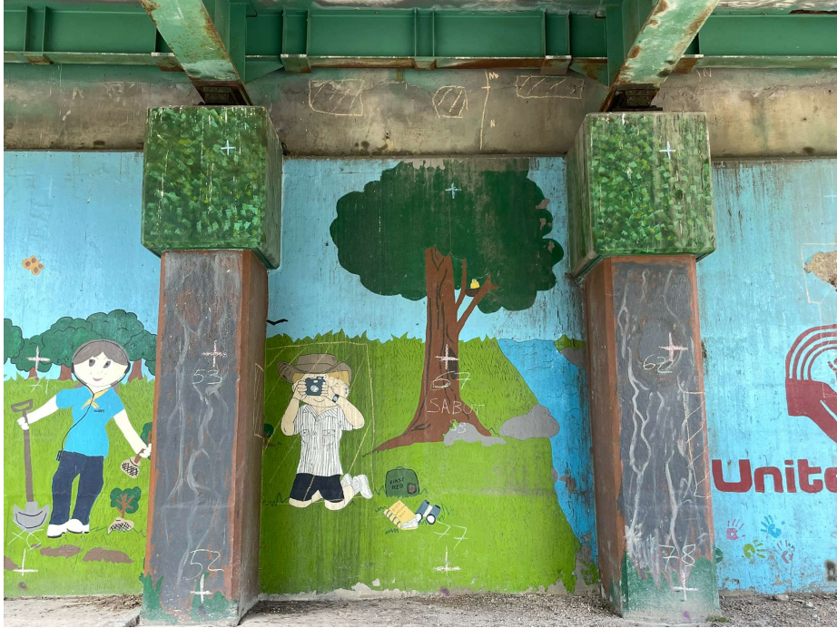
Photo 25 - South abutment wall, SB, between Column 8 and 9, large delamination and spalling near Column 8
