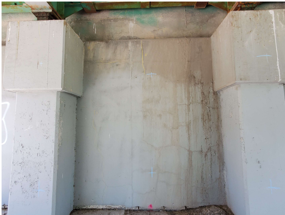
Photo 12 - North abutment Columns 8-9 (under NB lanes), joint leakage staining and narrow cracking in concrete refacing
