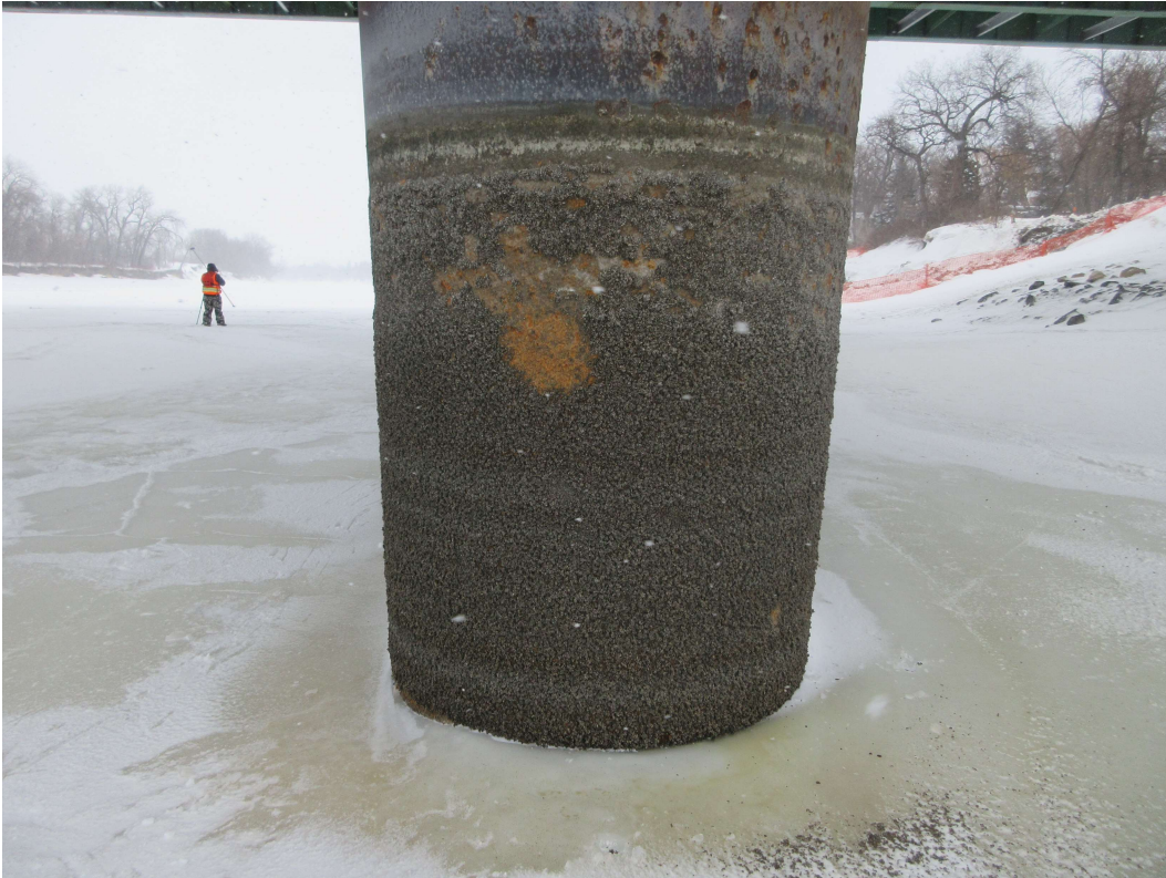
Photo 43 - Medium to Severe Pitting on Pier 6 Nosing
