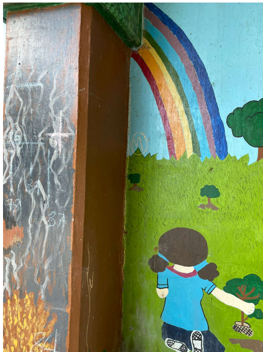
Photo 22 - South abutment wall, SB, near Column 7, medium cracking between column
