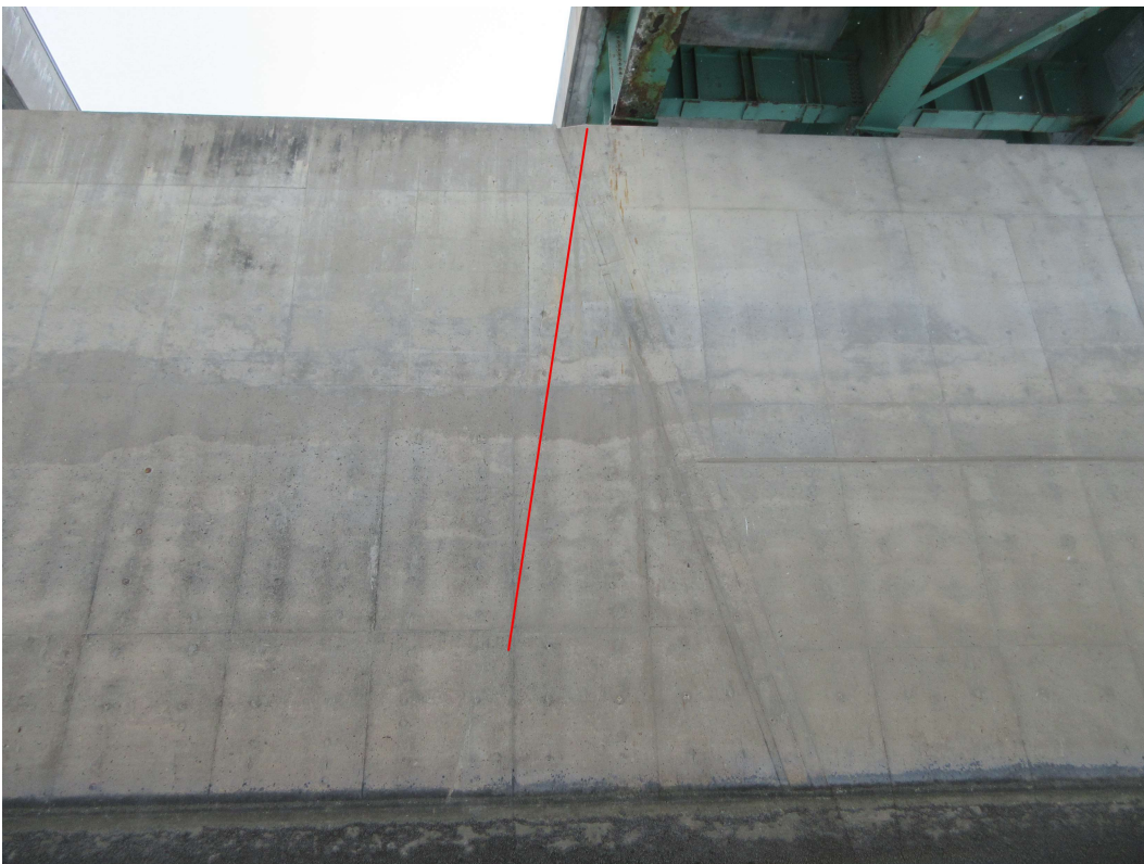
Photo 42 - Pier 5 South Face Medium Crack 21 of 22
