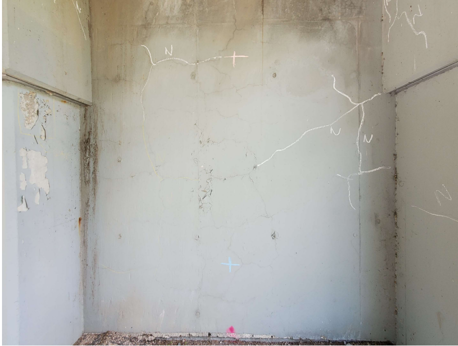
Photo 15 - North abutment wall refacing locations, narrow cracking is partially obscured by anti-graffiti coating
