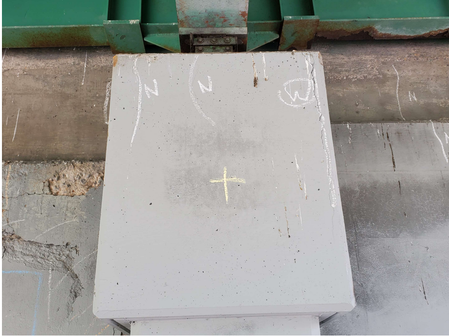
Photo 09 - North abutment wall, Column 3 cap south face, narrow to wide cracking
