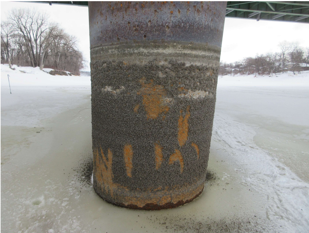
Photo 34 - Medium to Severe Pitting on Pier 4 Nosing 17 of 22
