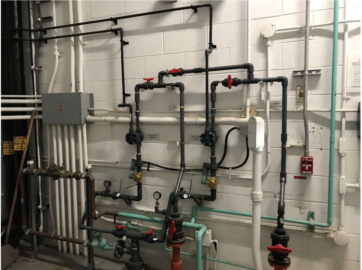
Photograph McP-1.4: McPhillips Chlorinator Room Looking at Educators
