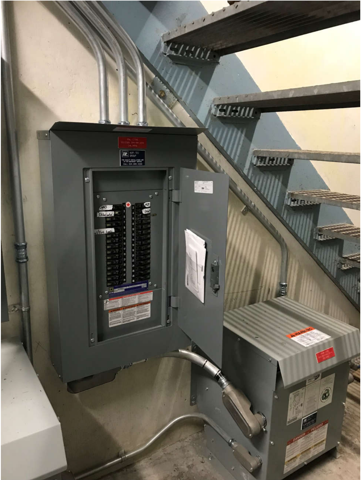
Photograph McP-1.9: McPhillips Chlorine 120/208V Standby Power
