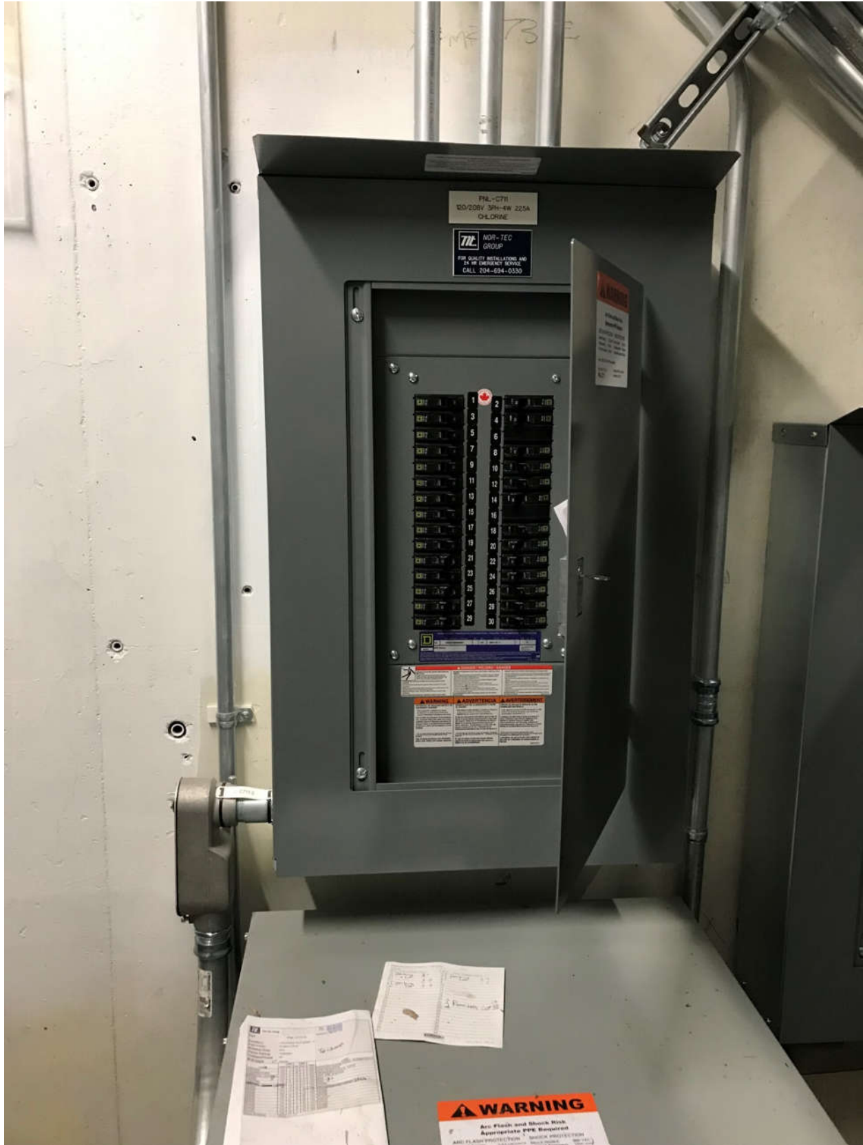
Photograph McP-1.8: McPhillips Chlorine Building 120/208V Normal Power
