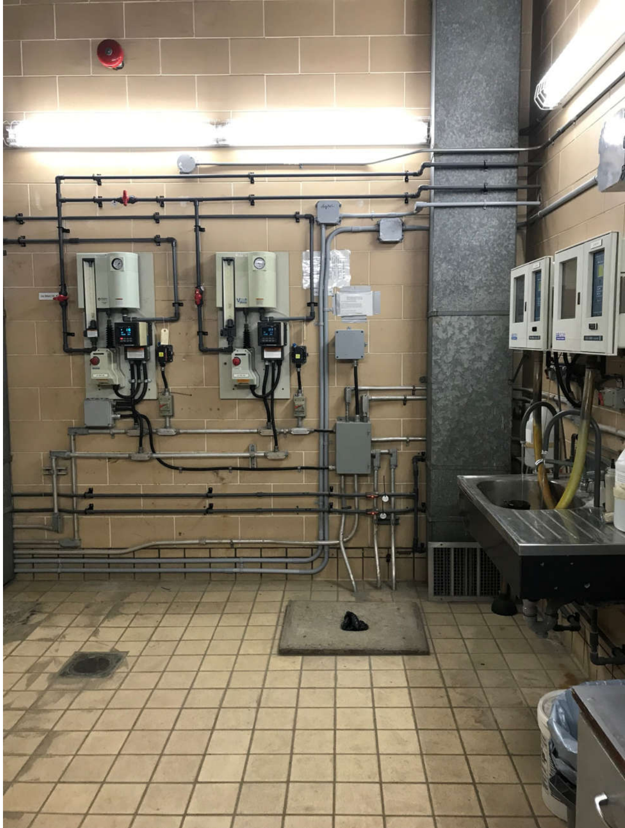
Photograph MacL-1.5: MacLean Chlorinator Room Looking East
