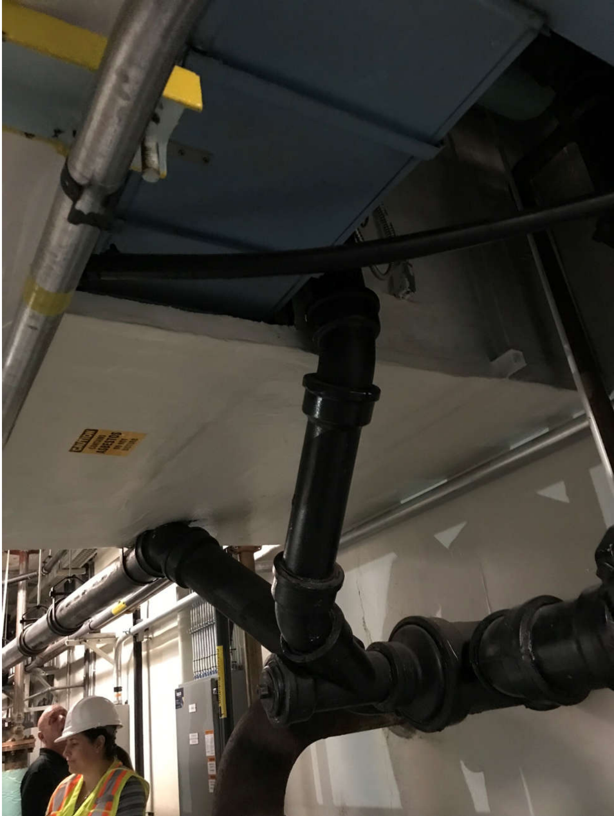
Photograph MacL-1.8: MacLean Mezzanine Level Below Ground Floor – Ventilation Air Riser Adjacent to Electrical Room
