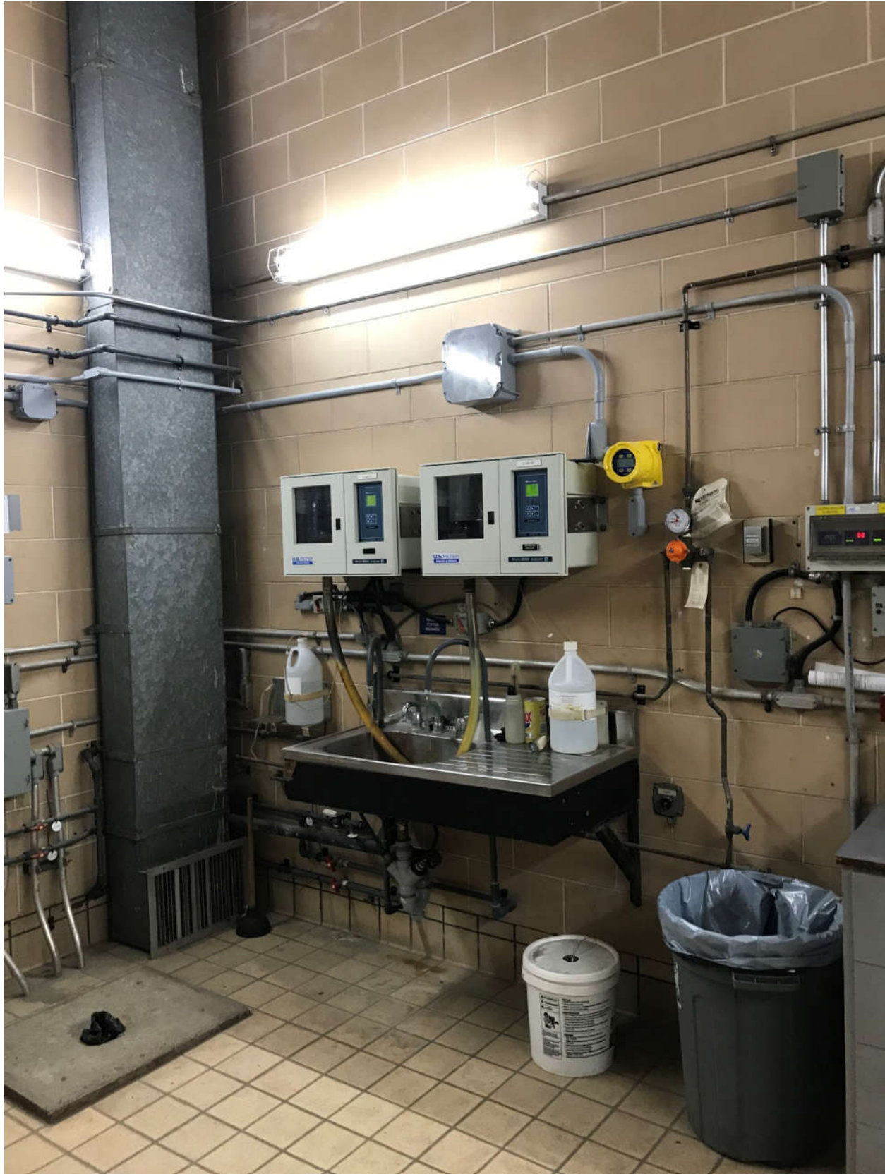
Photograph MacL-1.7: MacLean Chlorinator Room Looking South East
