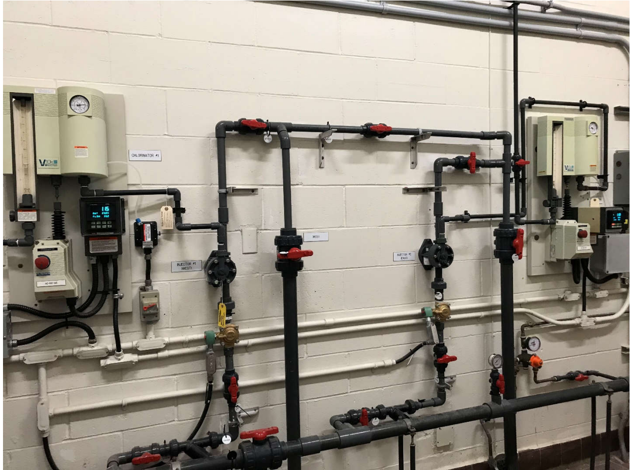
Photograph HUR-1.11: Hurst Chlorine Room Looking North
