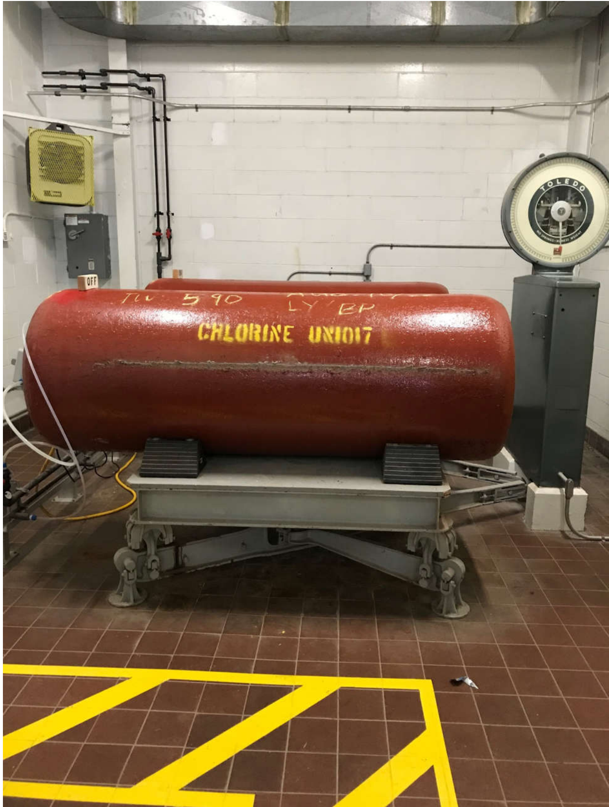
Photograph HUR-1.8: Hurst Tonner Chlorine Dosing Scales
