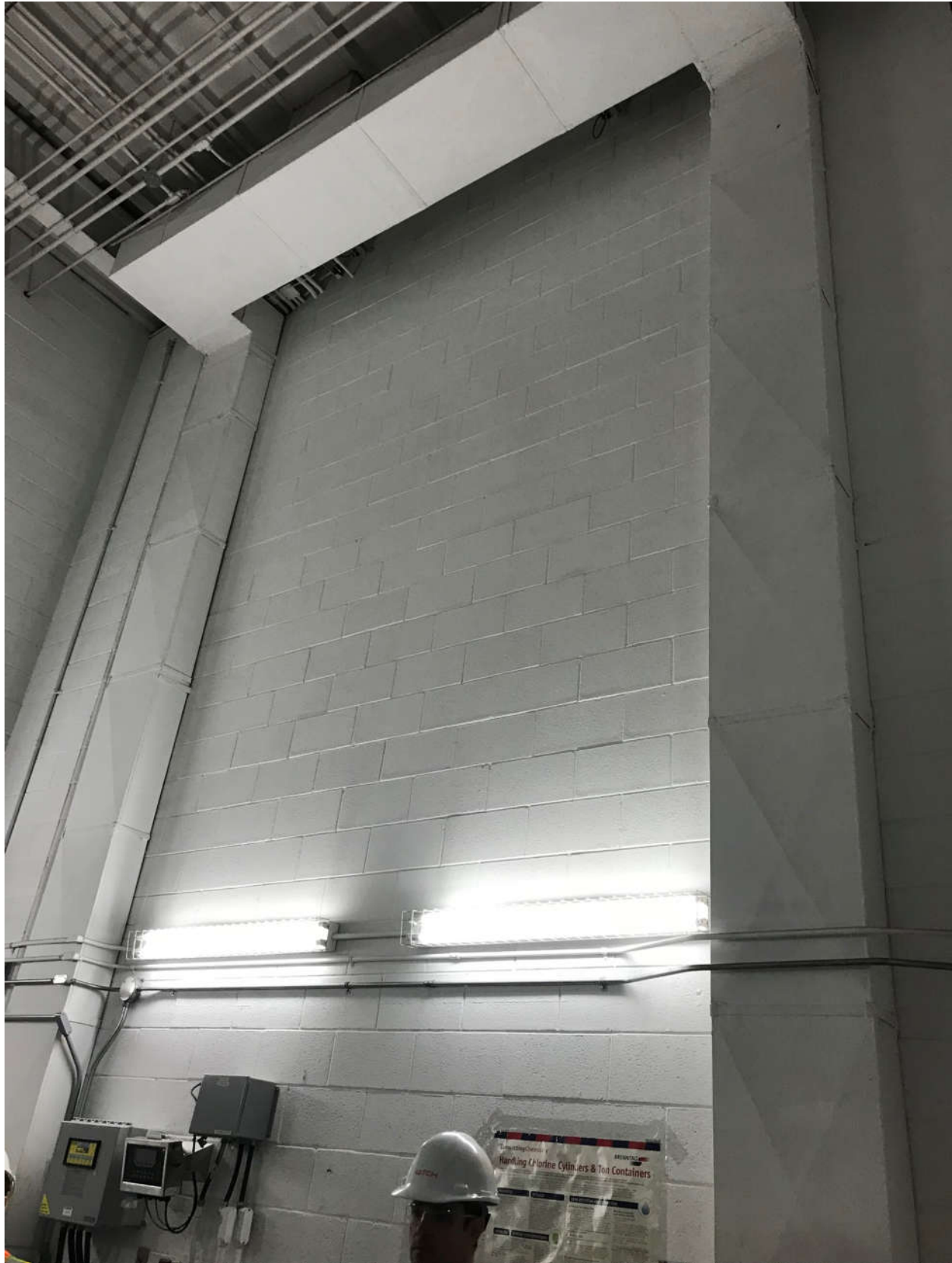
Photograph MacL-1.3: MacLean Tonner Room Chlorine Scale Area Exhaust Air Ducts
