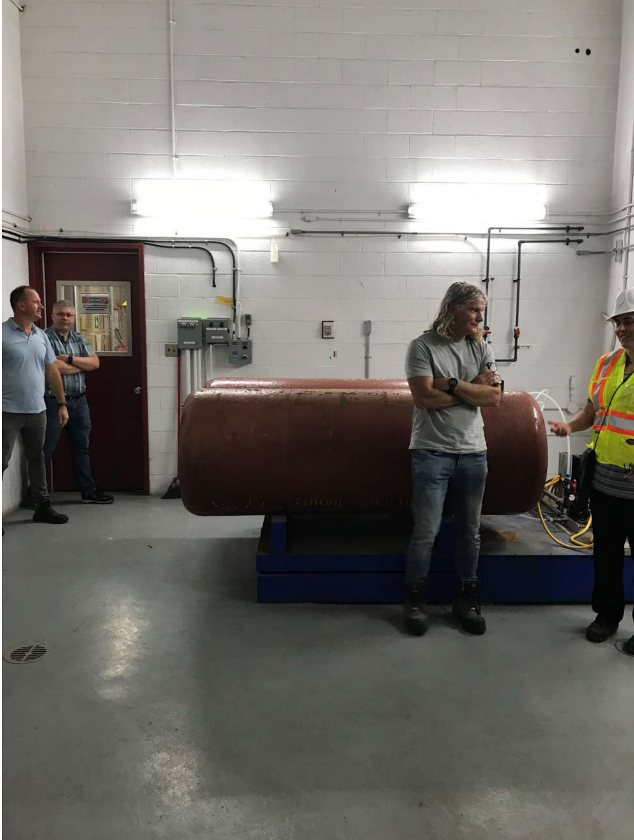
Photograph MacL-1.2: MacLean Tonner Room Chlorine Scales
