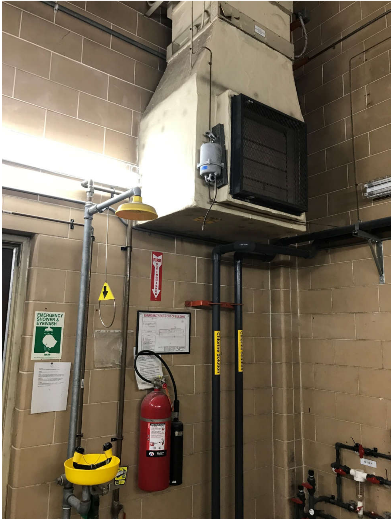
Photograph MacL-1.6: MacLean Chlorinator Room Outside/Return Air Duct and Heater
