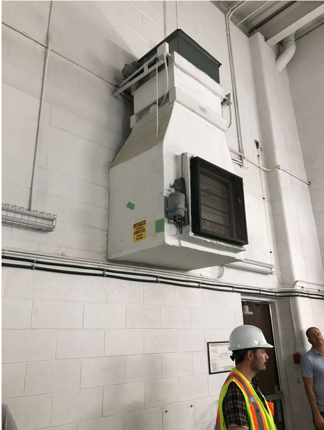
Photograph MacL-1.4: MacLean Tonner Room Chlorine Scale Area Outside/Return Air Duct and Heater
