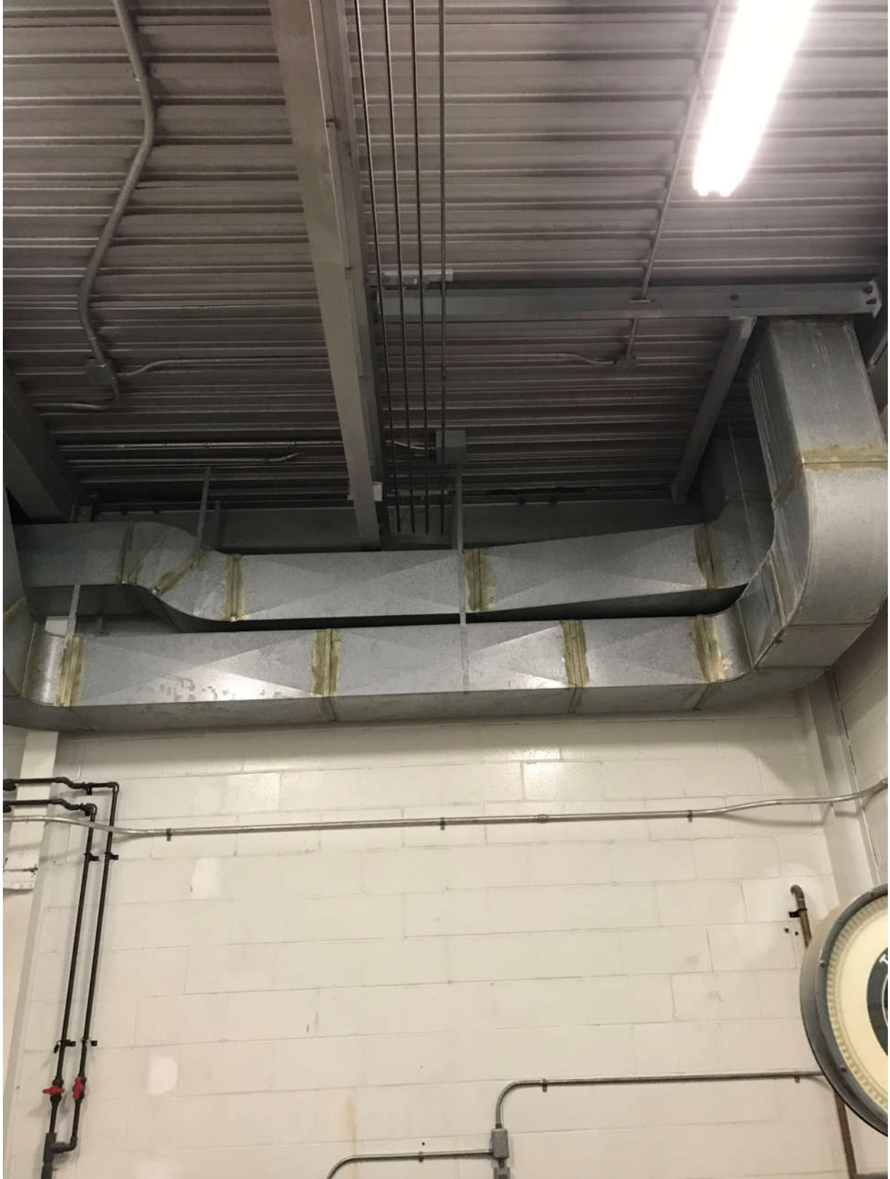
Photograph HUR-1.9: Hurst Tonner Scale Area and Chlorinator Room Ventilation Ducts
