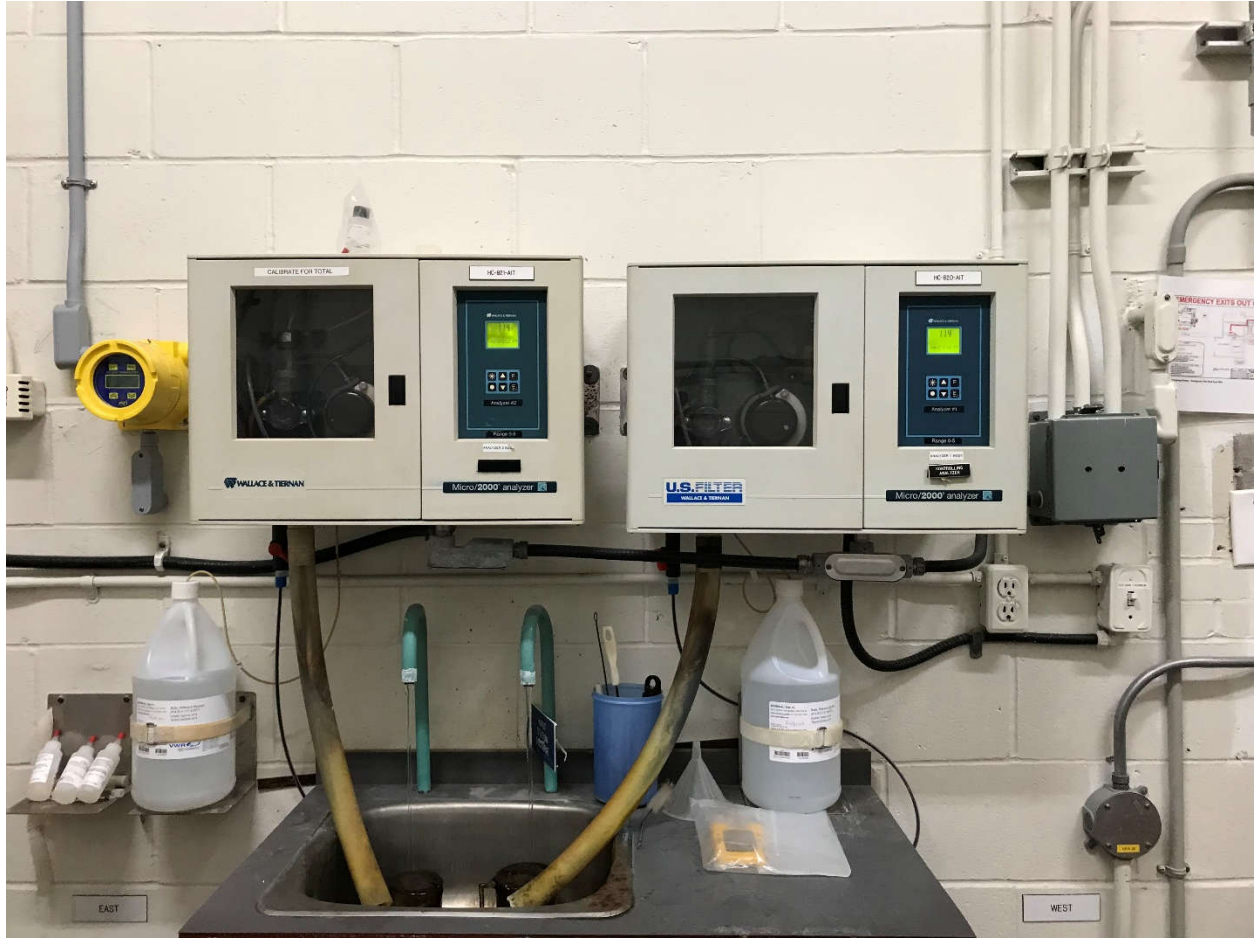
Photograph HUR-1.12: Hurst Chlorinators Room Looking South
