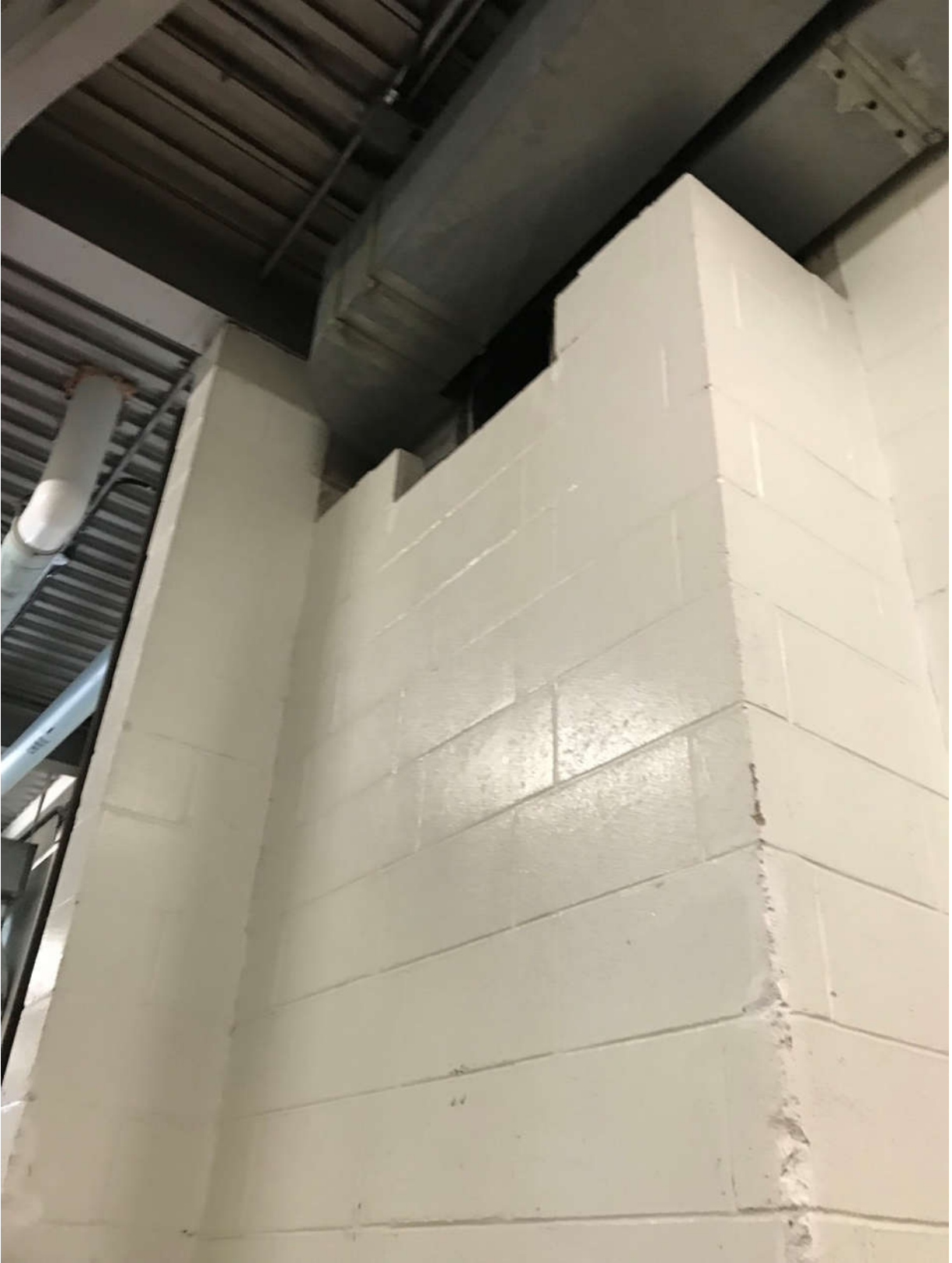
Photograph HUR-1.10: Hurst Tonner Scale Area and Chlorinator Room Ventilation Ducts and Wall Penetrations
