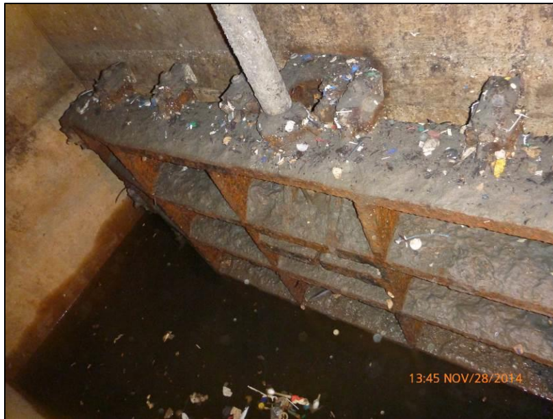
Photograph No. 9 Positive sluice gate
