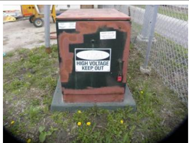
Photo #14 – View of padmounted transformer located near the northeast corner of the Public Works Yard.
