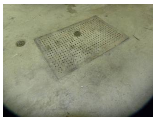
Photo #17 - View of floor drain located centrally in the main Public Works building.
