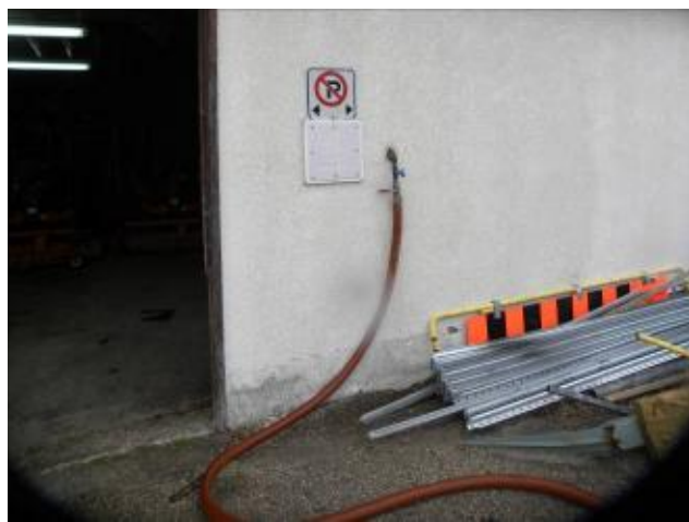
Photo #23 – View of chemical fill station located near the southeast corner of the main Public Works building.
