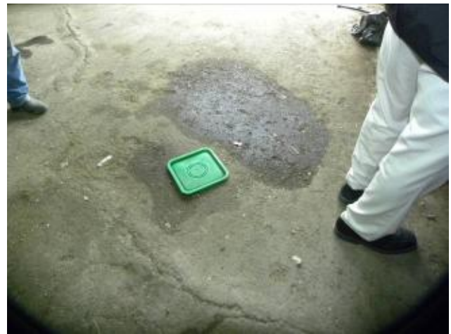
Photo #16 – View of dark staining on concrete flooring within the main Public Works building. Note cracking and pitting.
