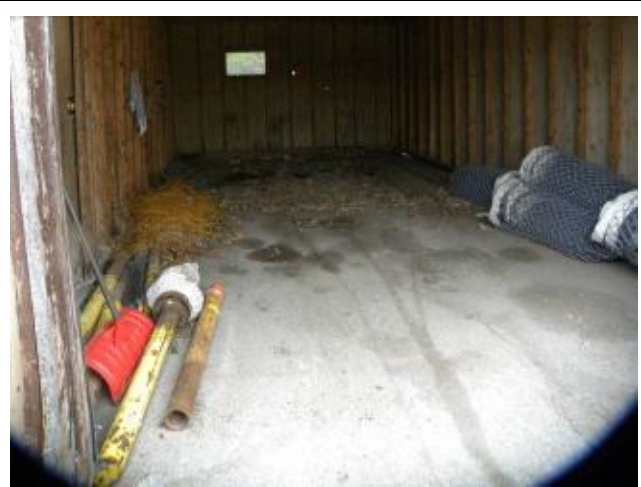
Photo #6 – View of interior of second storage shed at Public Works Yard. Note dark staining on asphalt surface.
