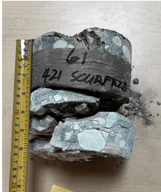
Scurfield Blvd, SBL ++ , Core 61 (Concrete Thk 140mm)
