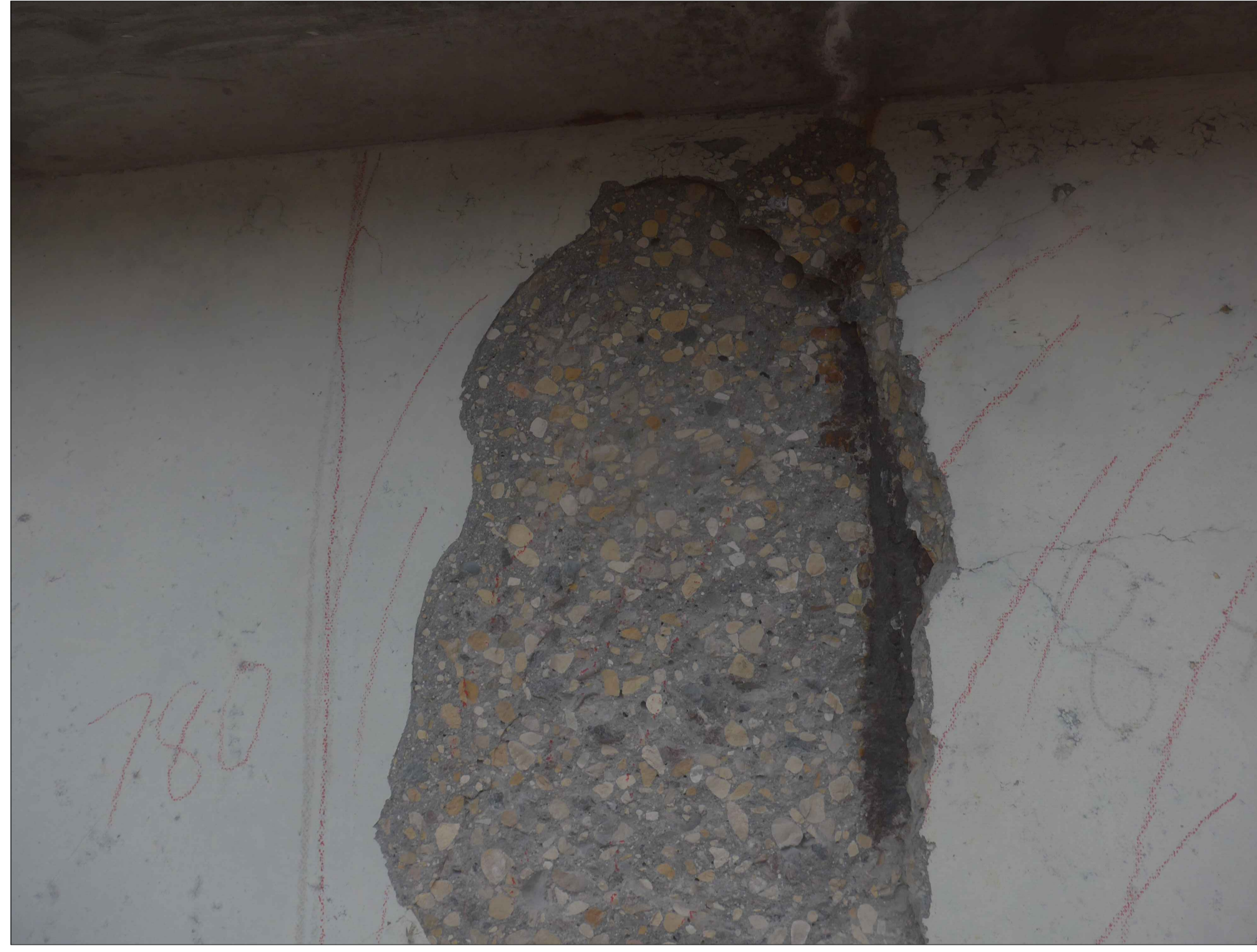
TYPICAL DELAMINATION ON NORTHBOUND BRIDGE SPANDREL WALL
