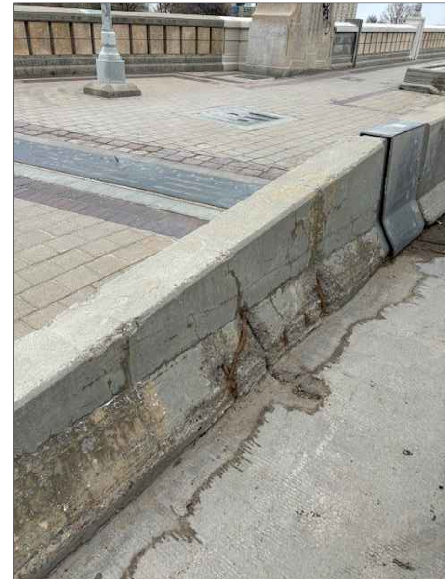
PHOTO 2 - NE CONCRETE BARRIER REPAIR AREA
