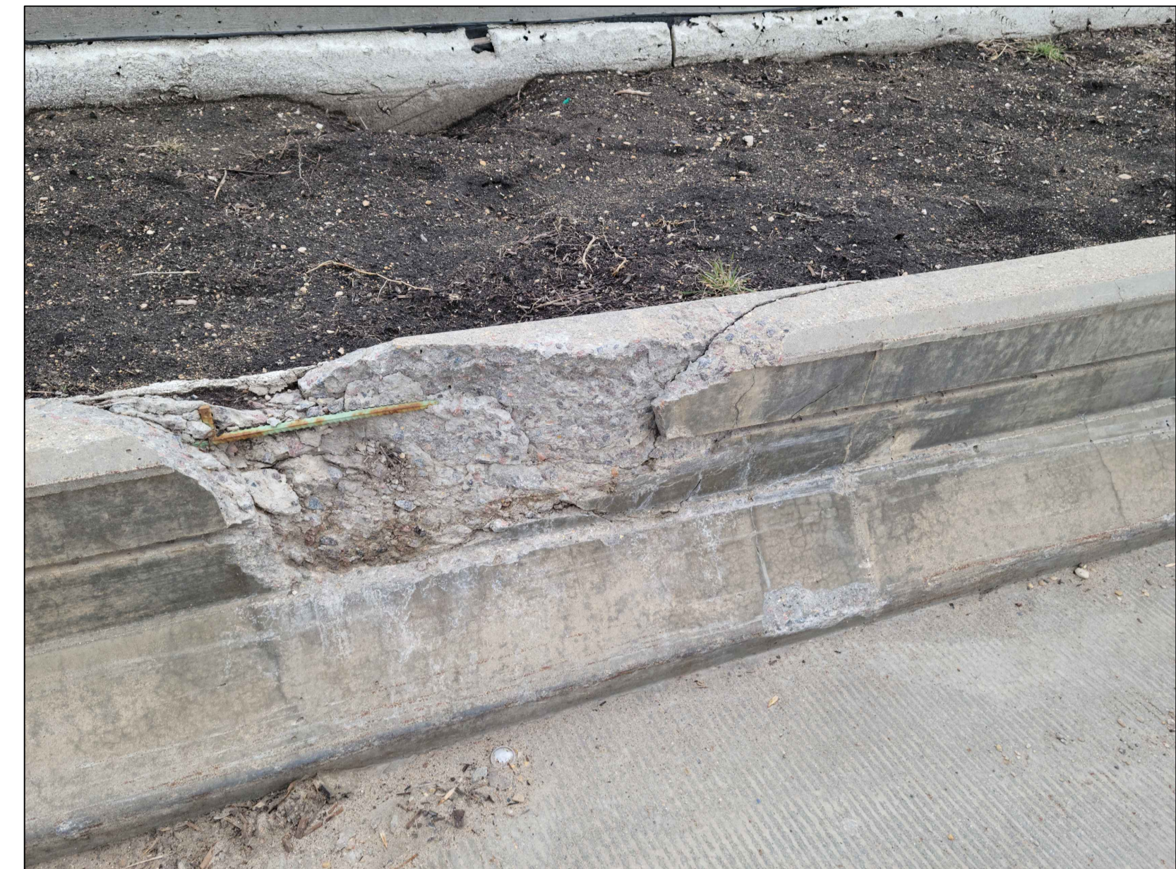
PHOTO 1 - PRECAST PLANTER WALL REPAIR AREA
