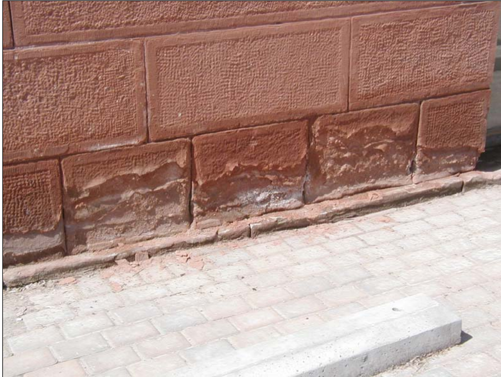
Plate 32 – Deterioration of the sandstone at grade, east side of building. ( M. Peterson, 2003. )
